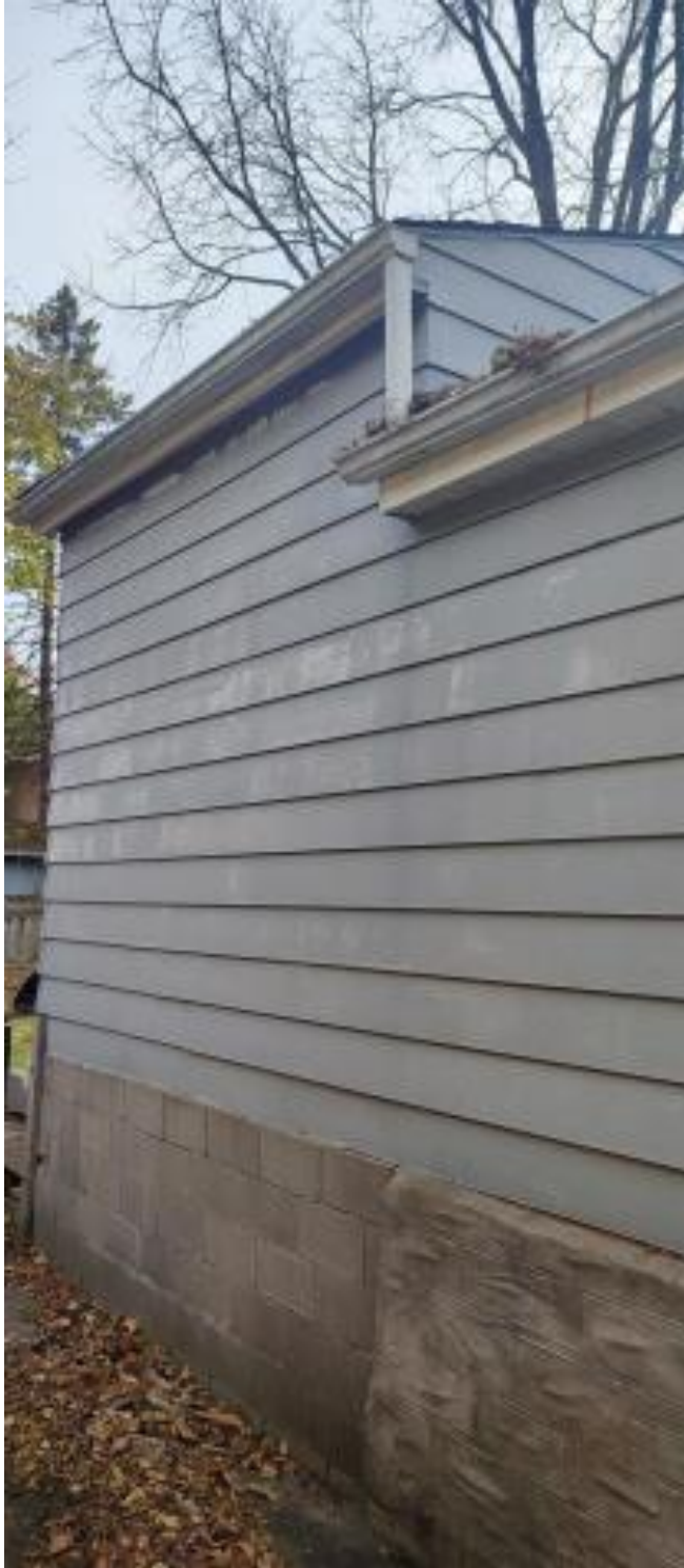
Figure 3: East elevation of the residential dwelling showing the addition proposed for removal (note cinder block foundation and raised roof)
