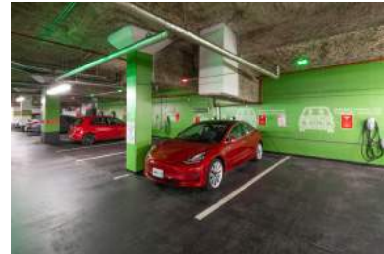
Level 2 and Tesla electric vehicle charging stations
