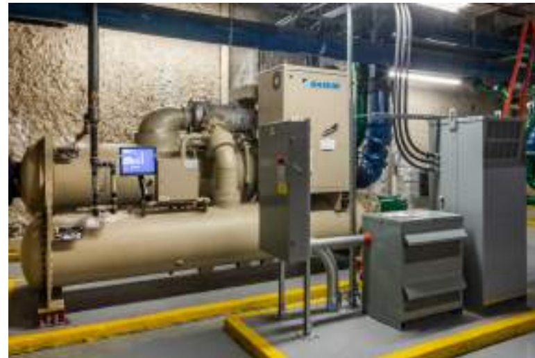
Ice Storage Cooling System to reduce power consumption
