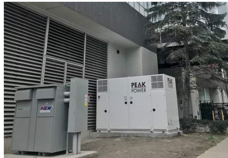
Offsetting Peak Power Demands by using an energy storage system
