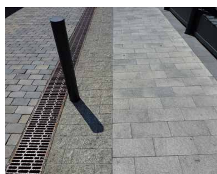
Figure 102 Precedents: Unique bollard elements may define areas for vehicles, with other forms of demarcation including mountable curbs and urban braille communicating transitions between zones.
