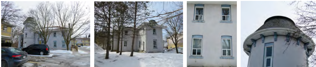
HERITAGE LISTED BUILDING – converted to apartments in 1991 by the current owner – industrial spray stucco applied to the masonry is in poor condition – the only original elements are the slate roof on the tower and some wood brackets that date from the 1860s
