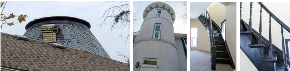
CURRENT CONDITIONS – the 1840s frame portion has not survived and there is a 1991 addition in this location that contains a stairwell and elevator that is not in service - the exterior masonry has been coated with a cement stucco that is in poor condition – the original wood doors have been replaced and the original 2 over 2 wood windows have been replaced with vinyl windows – the only original exterior feature is the slate roof on the tower and some of the decorative wood brackets below the tower eaves - the interior has been reconfigured and original features and finishes have been removed with the exception of a curved wood staircase between the 2 nd & 3 rd floor of the tower
