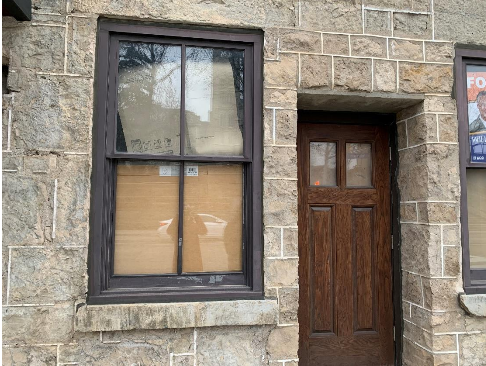
Figure 5 - 49 Norfolk St, entrance off Norfolk Street, right of main entrance (facing northeast) (Photo 2023 - V. Nagy)
