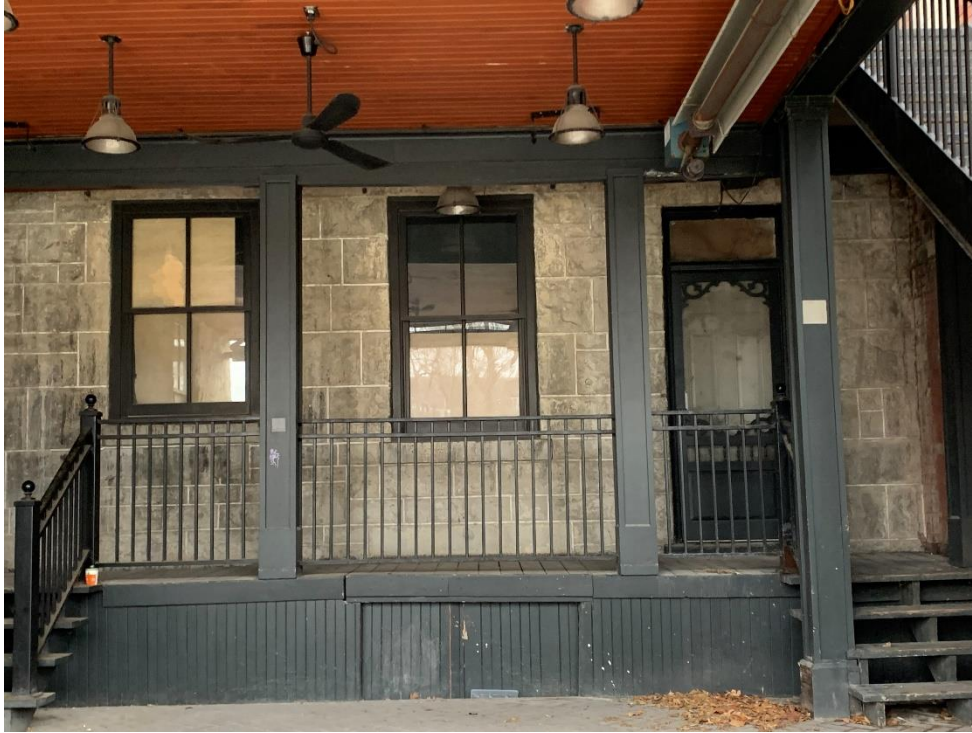
Figure 7 – Underneath modern balcony attached to east wall of 49 Norfolk Street (facing northwest) (Photo 2023 – V. Nagy)
