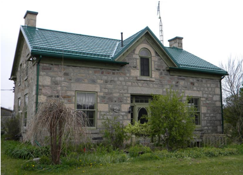
Attachment-3 Photos before boarding of windows and doors - 2010 (S. Robinson, Heritage Planning)
