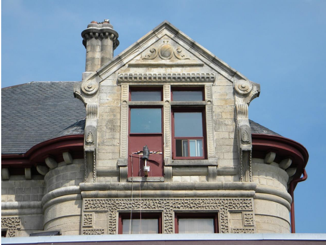
Figure 5 - 211 Silvercreek Parkway South, stone work present on the second storey and existing chimney (facing northwest) (Photo 2010 – S. Robinson)
