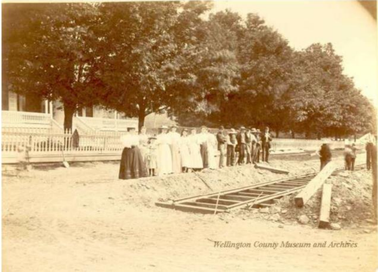
Figure 13 – Workmen laying streetcar tracks in front of the Sleeman House, c. 1900 (Wellington County Museum & Archives A1952.312.3B)
