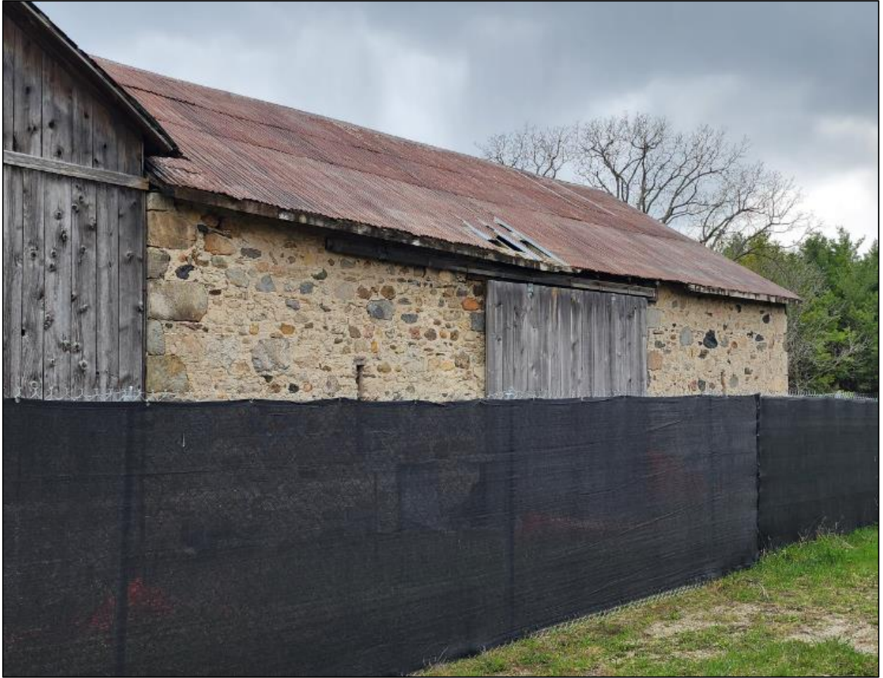
Figure 23: Photo of the barn entrance and temporary barrier. Taken April 25, 2023, by S. Robinson.
