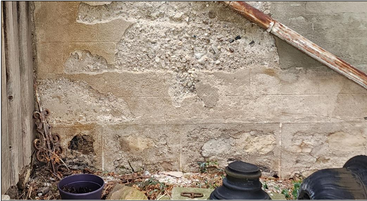
Figure 80: Photo of failing façade on exterior the farmhouse. Taken April 25, 2023, by S. Robinson.
