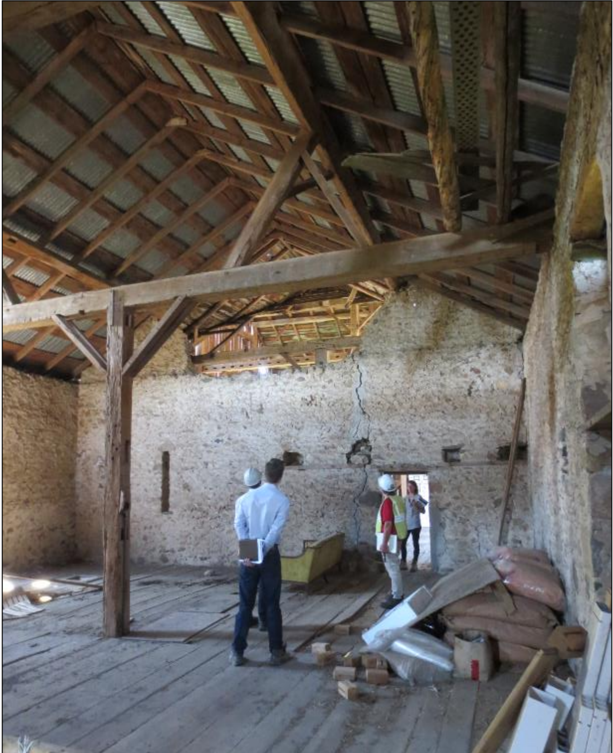
Figure 33: Photo of the stone barn's interior. Four people stand on either side of a large crack in the internal stone wall next to the internal doorway. Taken June 17, 2019, by S. Robinson.
