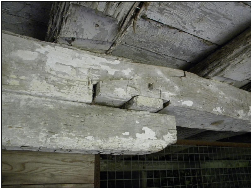
Figure 68: Photo of scarf joint in stone barn basement framing. Taken August 15, 2011, by S. Robinson.
