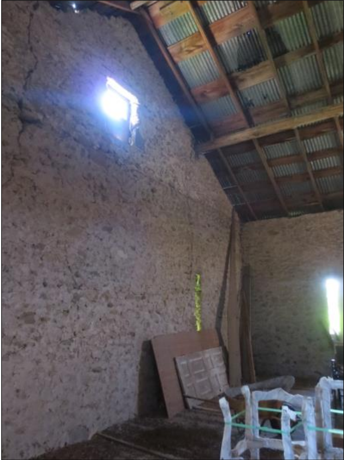
Figure 31: Photo of the barn's interior and the metal roof. A crack can be seen in the upper left corner. Taken June 17, 2019, by S. Robinson.
