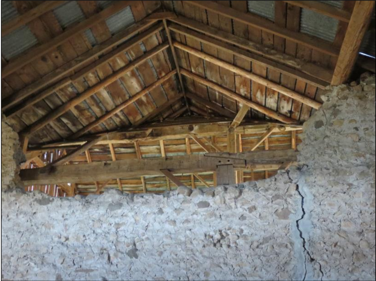
Figure 35: Photo of the section removed from the barn's interior wall. The ceiling of the wooden addition is visible through the space, and a crack is visible down the wall to the right. Taken June 17, 2019, by S. Robinson.
