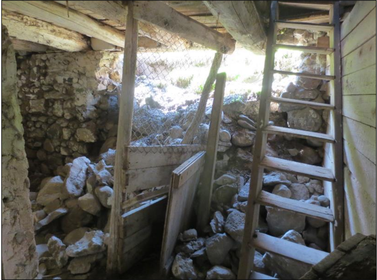
Figure 46: Photo of root cellar, showing the collapsed section of foundation. Taken June 17, 2019, by S. Robinson.
