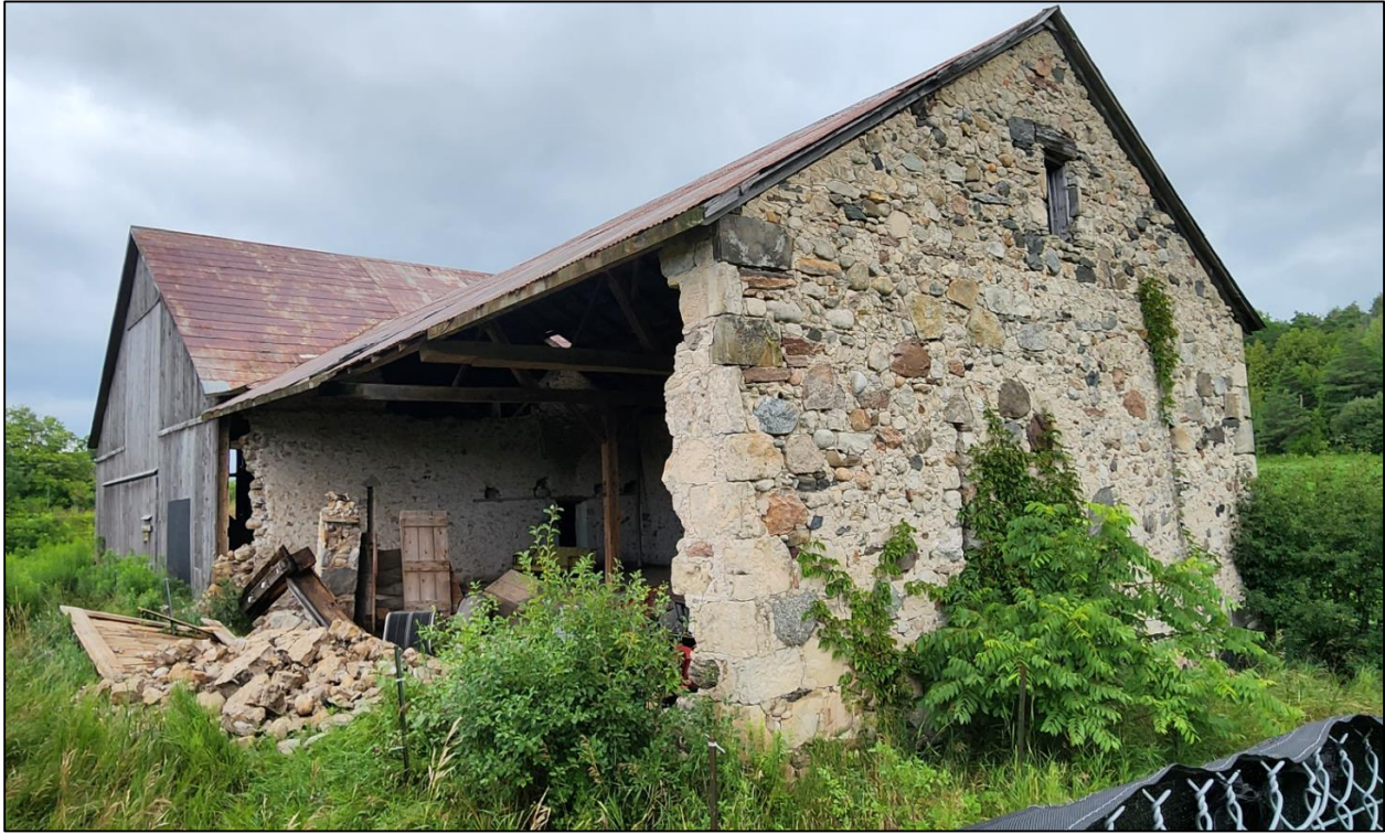
Figure 10: Photo of collapsed barn wall. Taken July 27, 2023, by S. Robinson.
