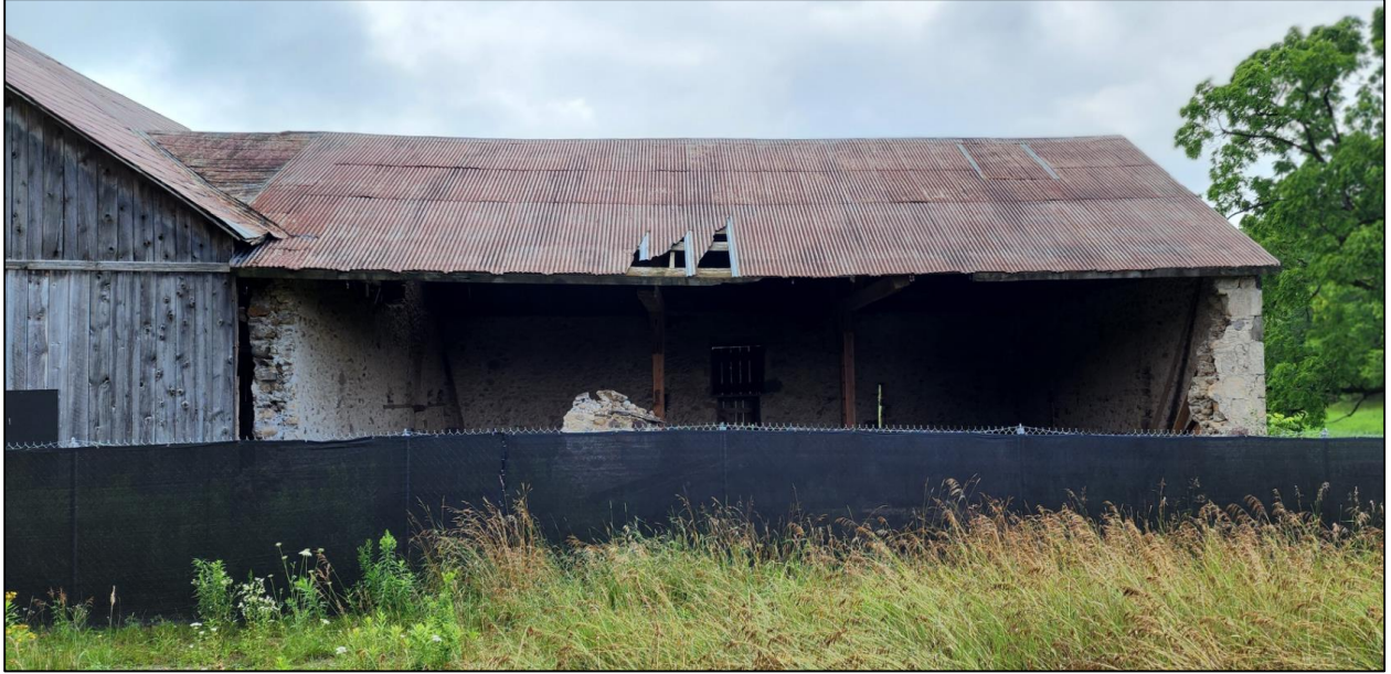
Figure 7: Photo of collapsed barn wall. Taken July 27, 2023, by S. Robinson.
