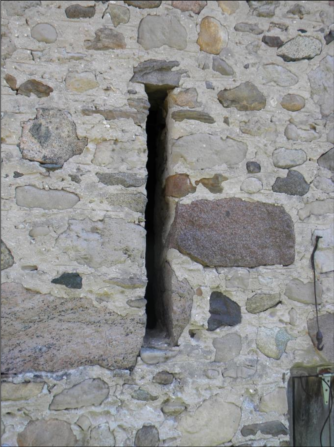
Figure 53: Photo of the stone barn exterior highlighting a compromised corner. Taken August 15, 2011, by S. Robinson.
