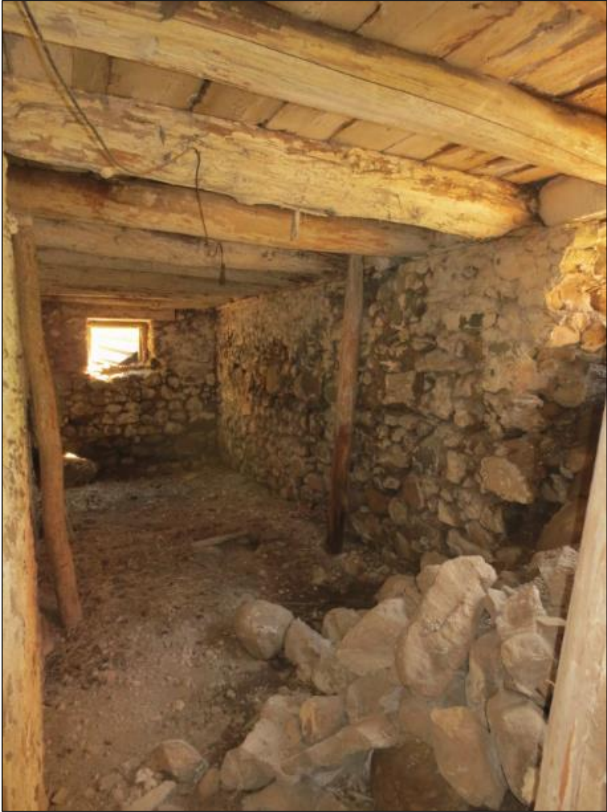
Figure 45: Photo of stone rubble in the basement of the stone barn. Taken June 17, 2019, by S. Robinson.
