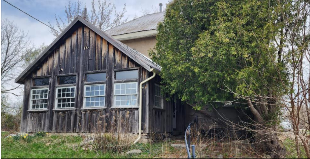
Figure 79: Photo of exterior of the rear extension of the farmhouse. Taken April 25, 2023, by S. Robinson.
