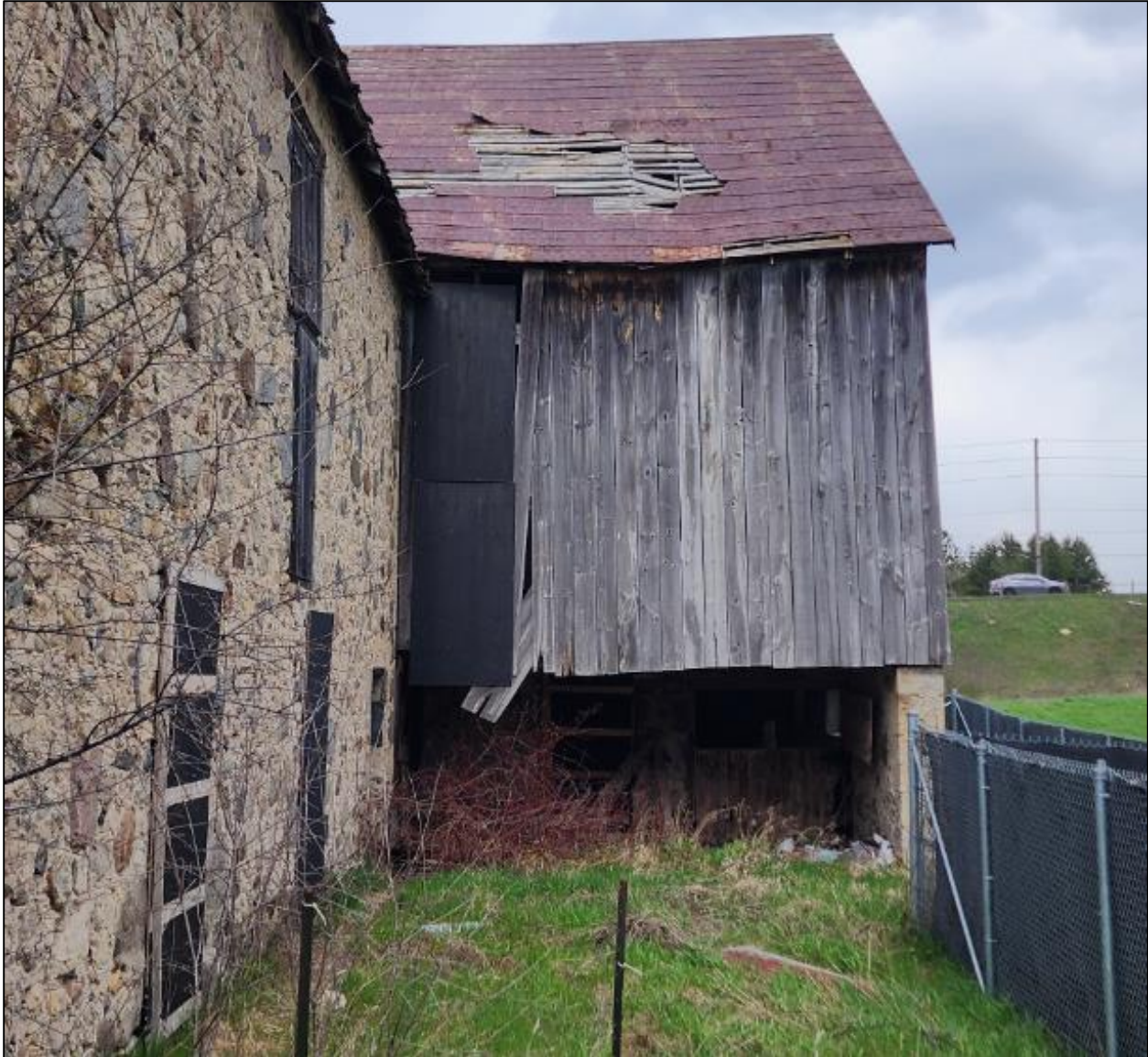
Figure 20: Photo of stone slot barn and wooden addition. Taken April 25, 2023, by S. Robinson.
