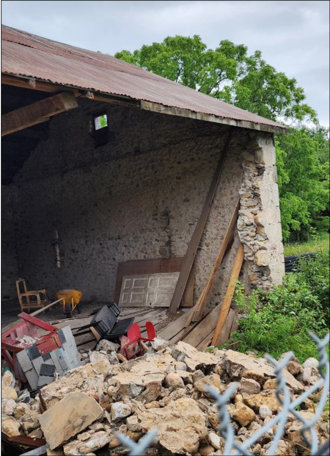
Figure 15: Photo of collapsed barn wall and interior with rubble in the foreground. Taken July 27, 2023, by S. Robinson.
