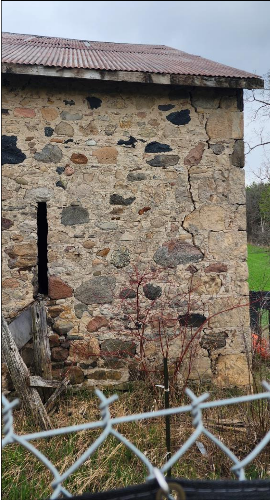
Figure 24: Photo of a crack the barn's exterior corner. Taken April 25, 2023, by S. Robinson.
