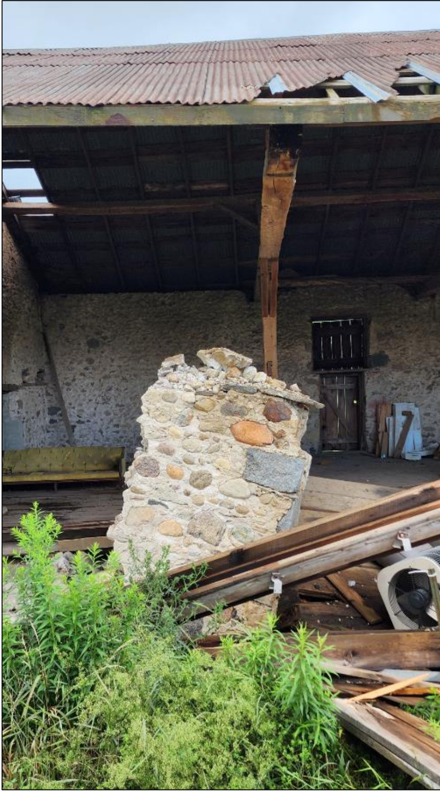
Figure 13: Photo of collapsed barn wall and barn interior. Taken July 27, 2023, by S. Robinson.
