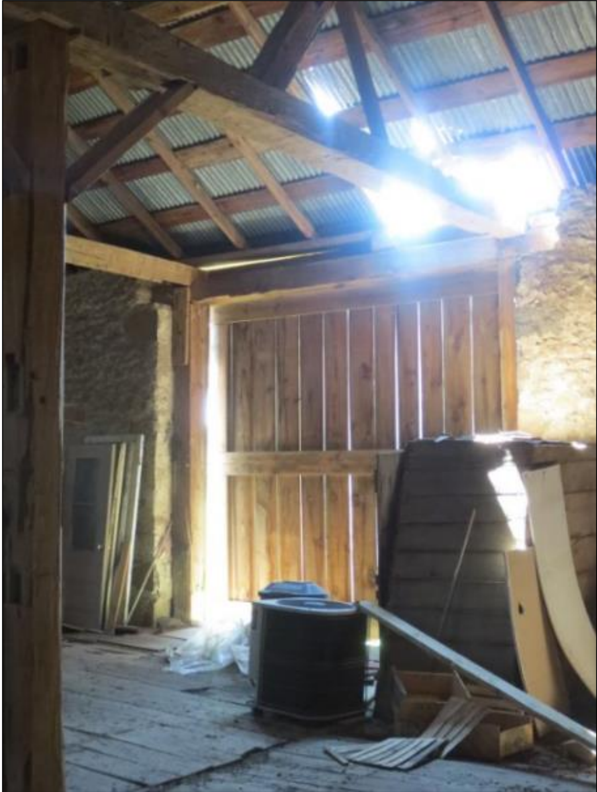
Figure 29: Photo of a hole in the roof above the main door. Taken June 17, 2019, by S. Robinson.
