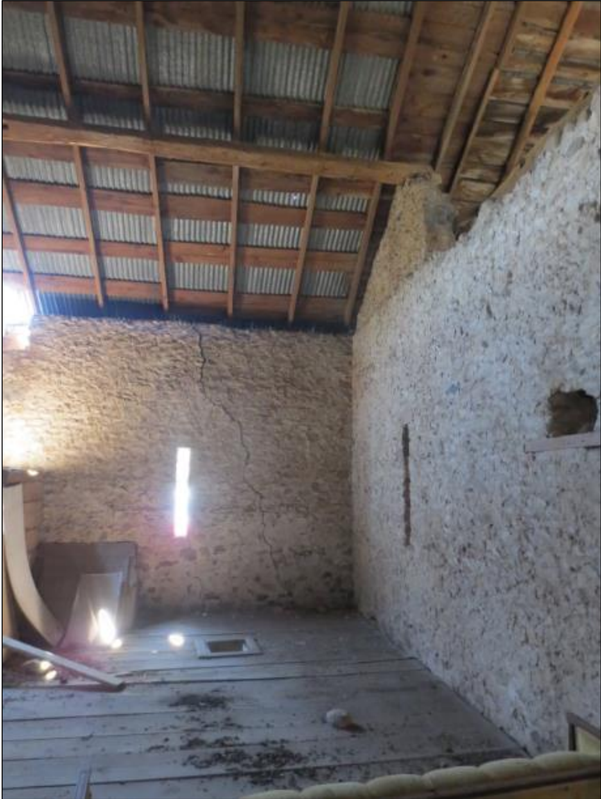
Figure 30: Photo of an internal crack in the exterior wall. Taken June 17, 2019, by S. Robinson.
