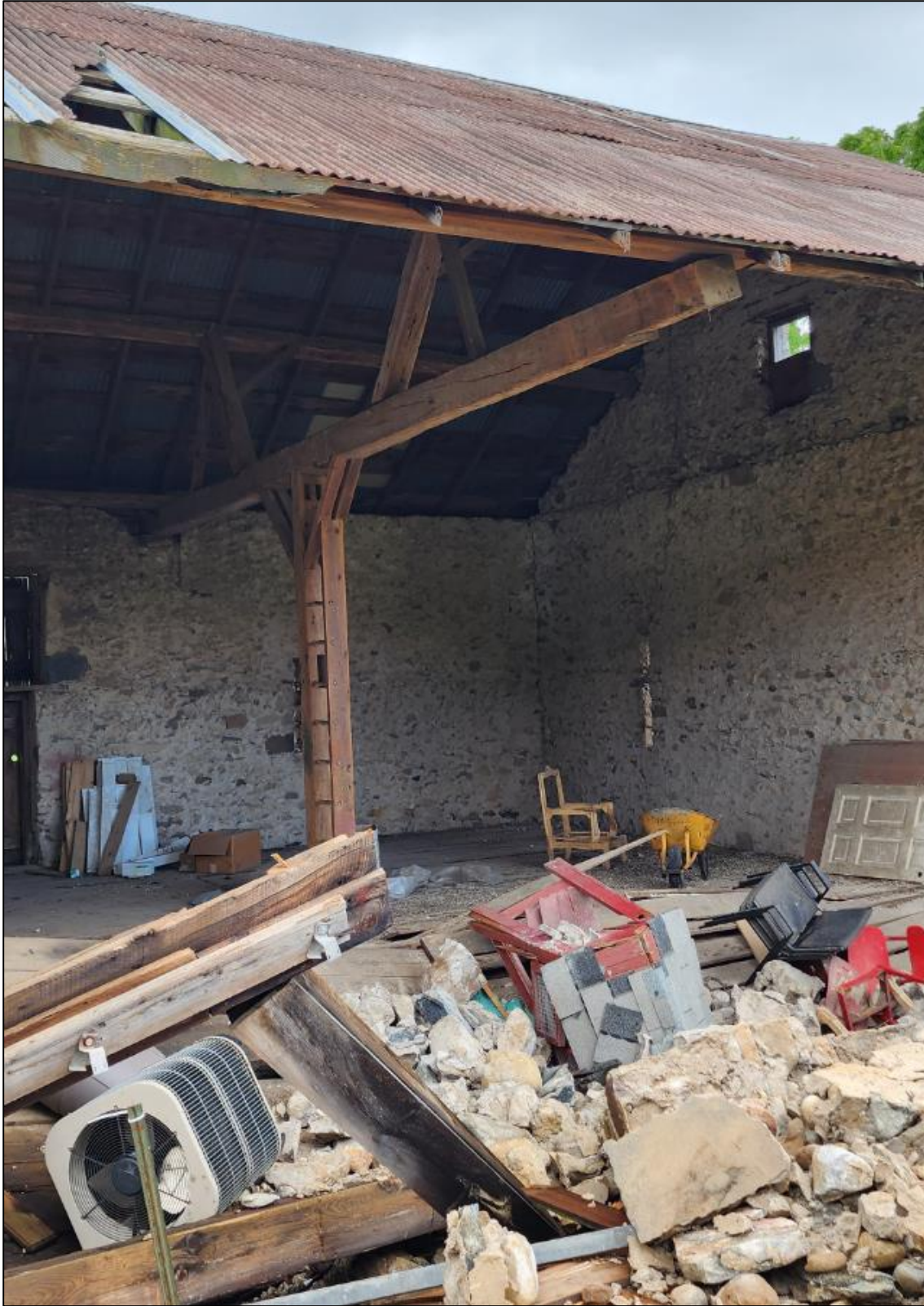
Figure 14: Photo of collapsed barn wall and interior. Taken July 27, 2023, by S. Robinson.
