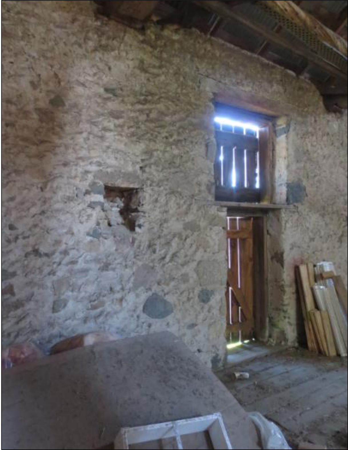
Figure 32: Photo of the barn's interior and pedestrian door. Taken June 17, 2019, by S. Robinson.
