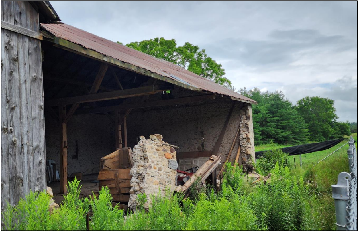
Figure 8: Photo of collapsed barn wall. Taken July 27, 2023, by S. Robinson.
