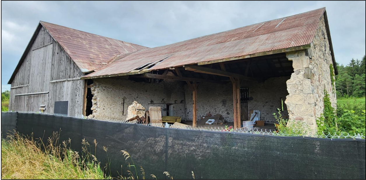
Figure 9: Photo of collapsed barn wall. Taken July 27, 2023, by S. Robinson.
