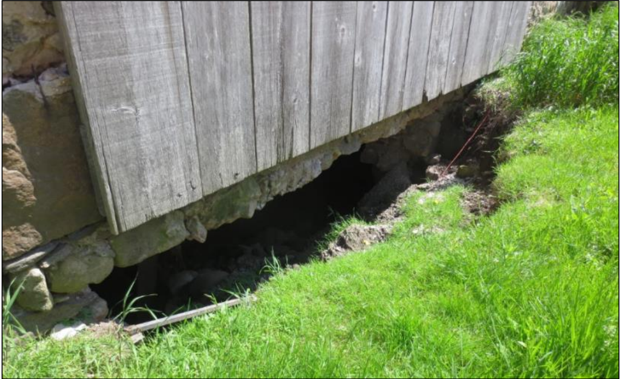
Figure 28: Photo of the barn's main door and failed foundation. Taken June 17, 2019, by S. Robinson.
