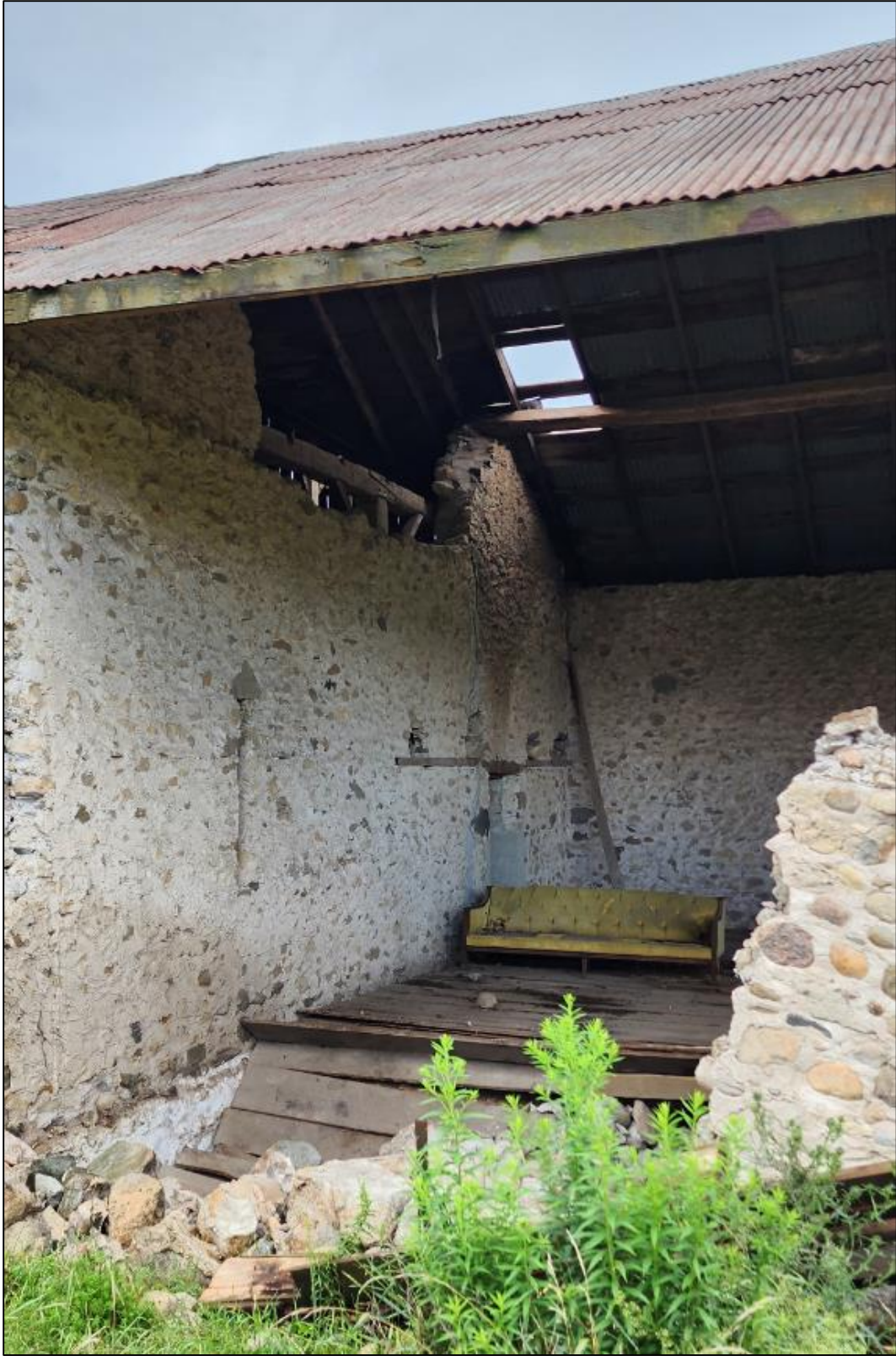
Figure 12: Photo of collapsed barn wall and interior of barn. Taken July 27, 2023, by S. Robinson.
