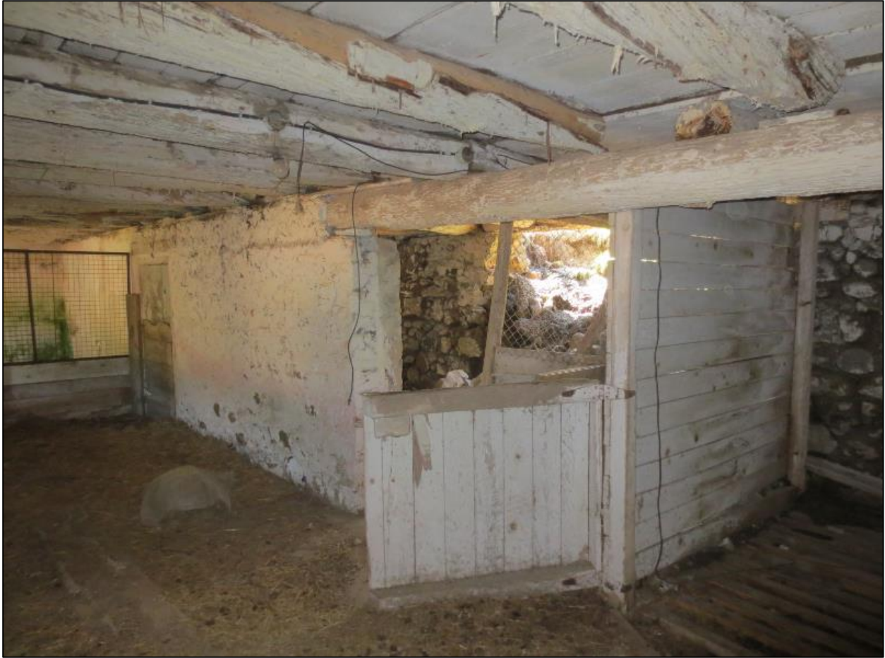
Figure 44: Photo of the root cellar and partially collapsed foundation. Taken June 17, 2019, by S. Robinson.
