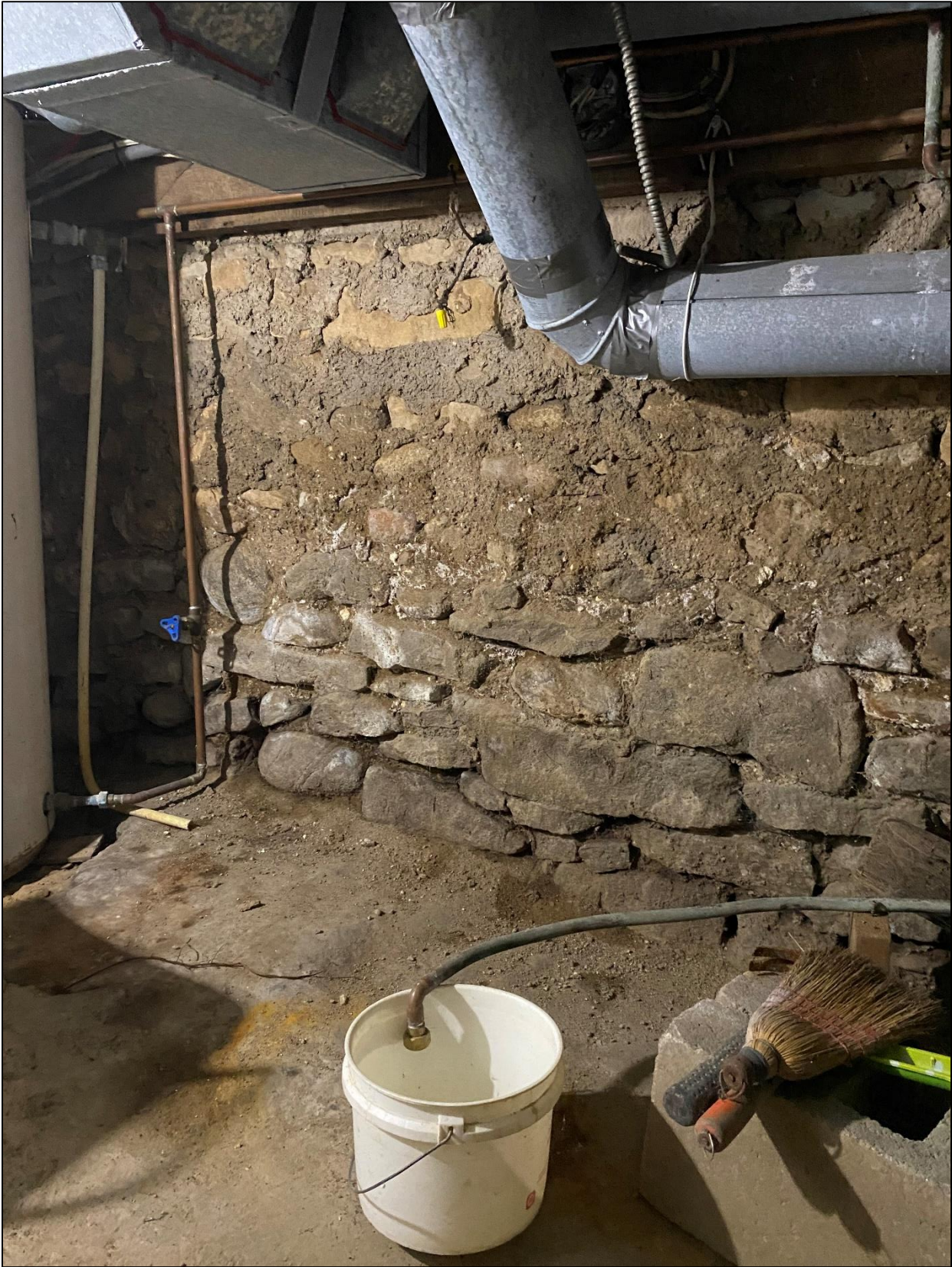
Figure 10: Stone interior wall in the basement
