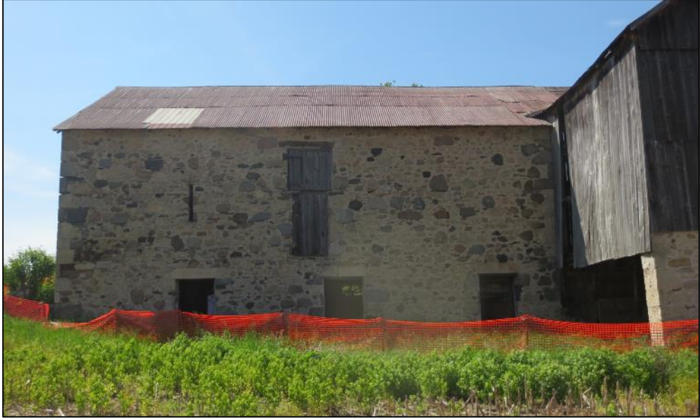
Figure 13: Photo of the stone barn's southern, 2-storey exterior. Taken June 17, 2019, by S. Robinson.
