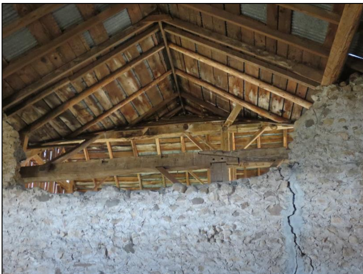
Figure 10: Photo of the upper section removed from the barn's east interior wall. The ceiling of the wooden addition is visible through the space. Taken June 17, 2019, by S. Robinson.
