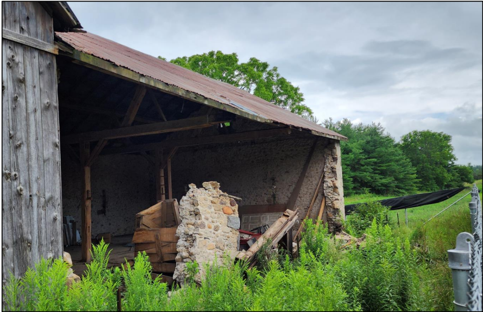
Figure 6: Photo of collapsed north stone wall. Taken July 27, 2023, by S. Robinson.
