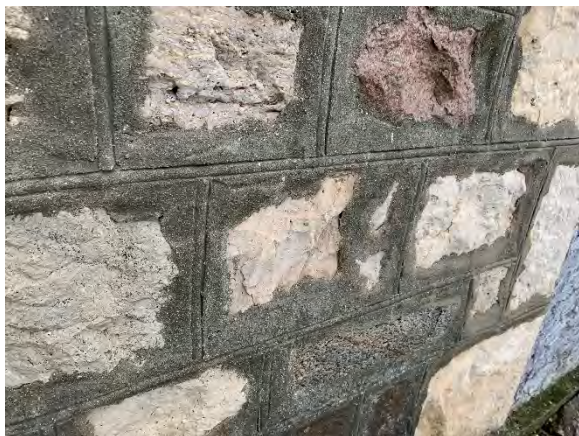
Photo 10: Typical Ashlar with Spalled Face and Tuck-pointing
