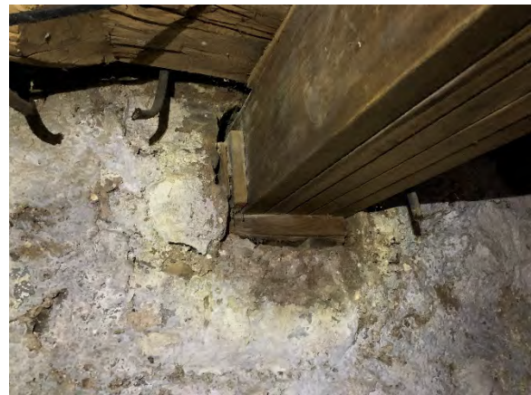
Photo 15: Typical Voids at Joist Ends
