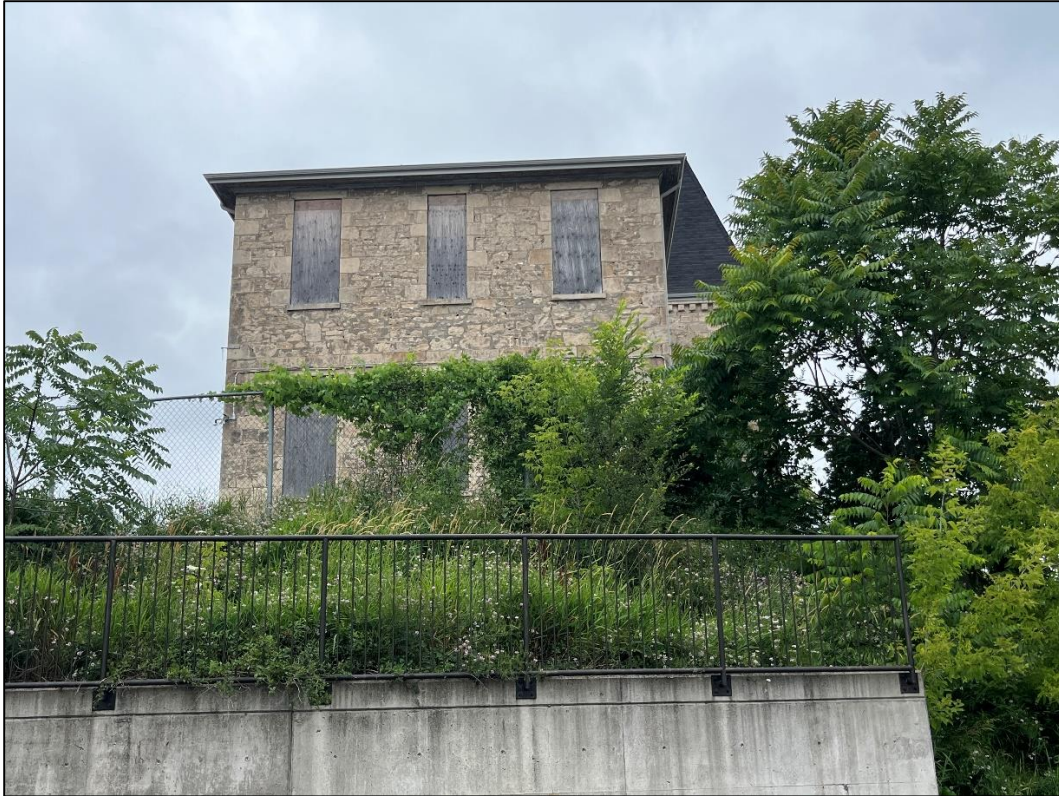
Figure 8: Northern façade of the building viewed from Guelph Civic Museum parking lot
