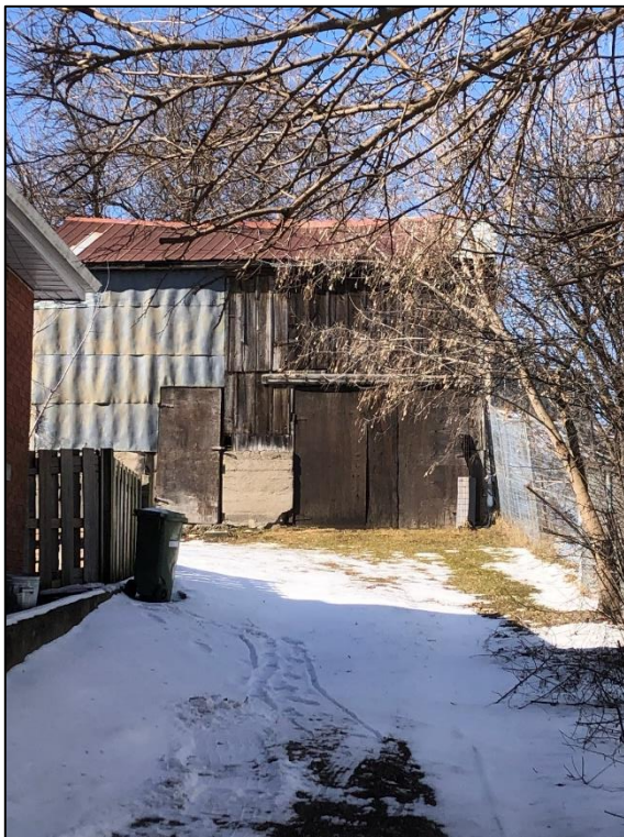
Figure 8: Photo of 14 Neeve barn taken from driveway on Surrey Street. Mixed materials for siding with red/rusting tin roof. Large sliding door on right side.
