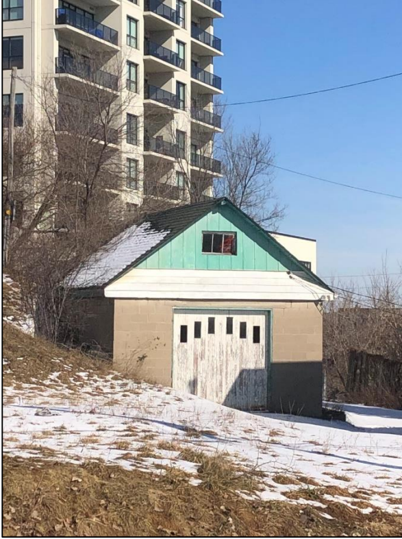
Figure 3: Photo of 14 Neeve Street garage. Stone walls, vinyl fascia, and a small window below the peak of a shingle roof.
