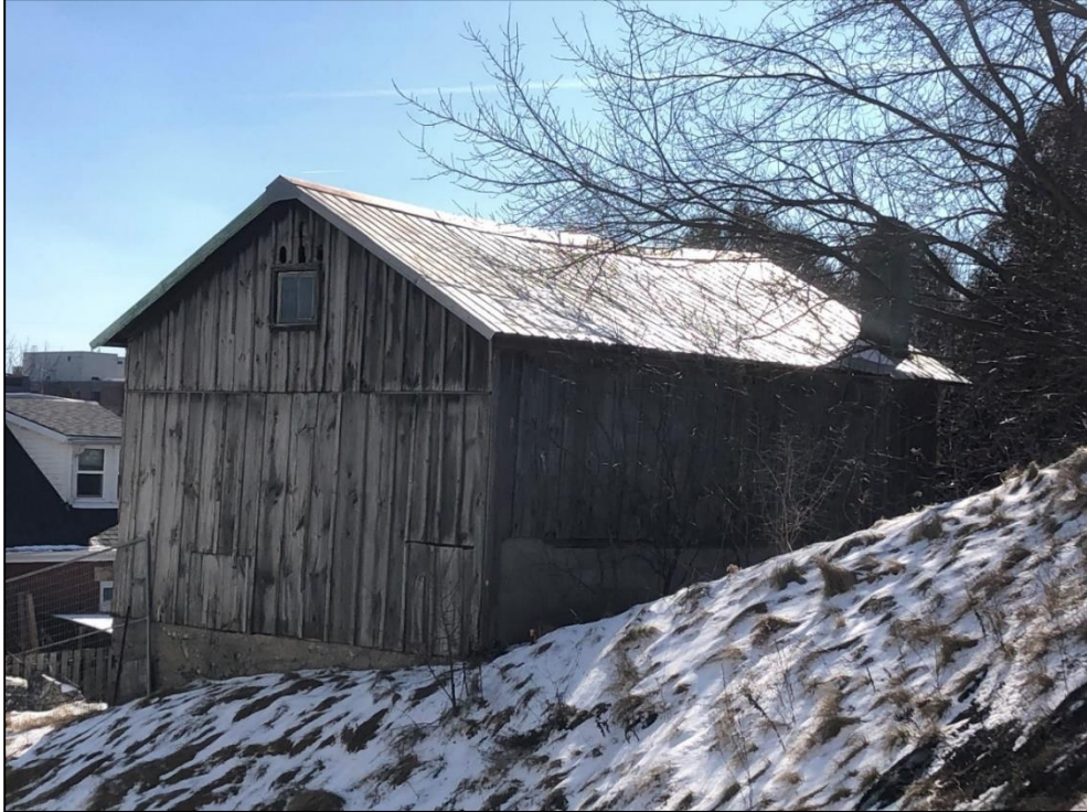
Figure 11: View of 14 Neeve Street barn from hill behind property. Tin roof and board and batten siding, with a stone chimney visible on right corner, partially obscured by trees.
