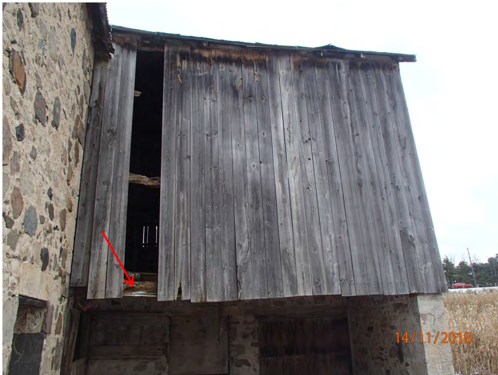
Photograph No. 15– Partially rotted floor beam, missing wall boards
