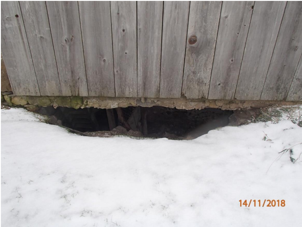
Photograph No. 1 – Foundation wall condition in 2018
