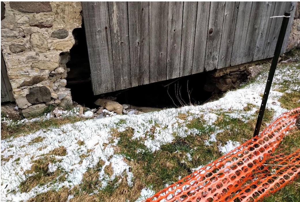
Photograph No. 2 – Foundation wall condition in 2021
