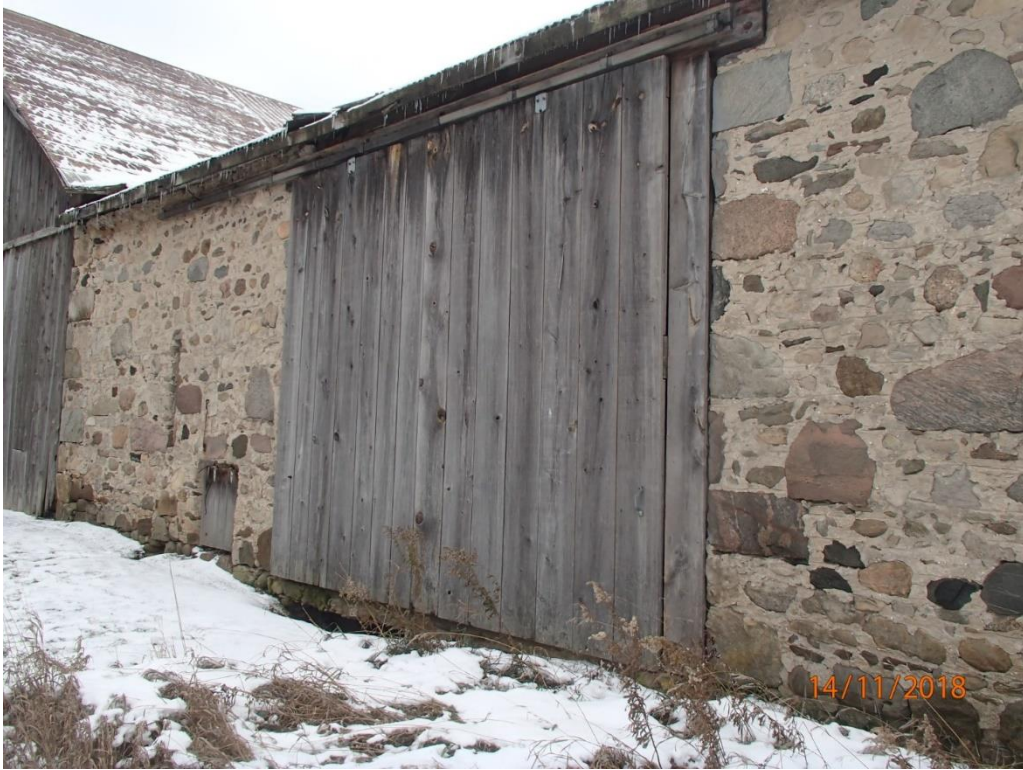
Photograph No. 7 – North Stone Wall (upper) condition in 2018
