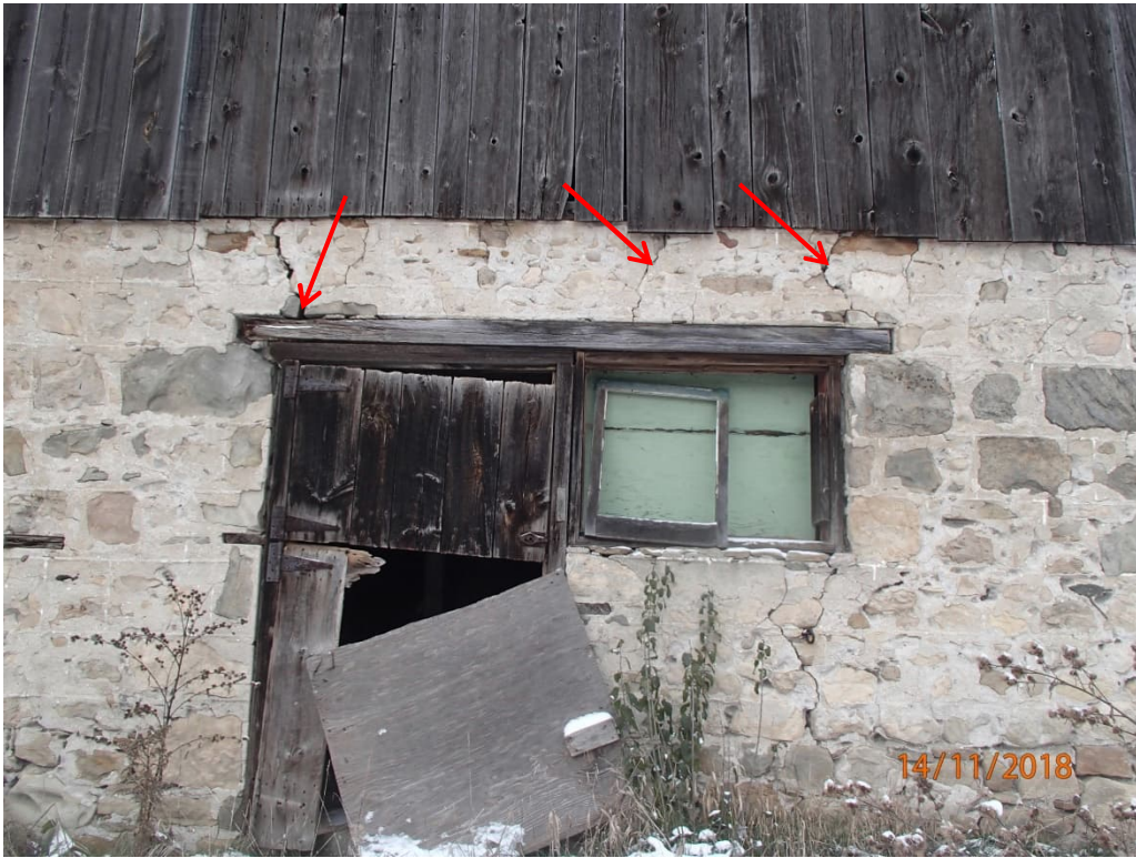
Photograph No. 17 – South wall, cracked stone over wood lintel
