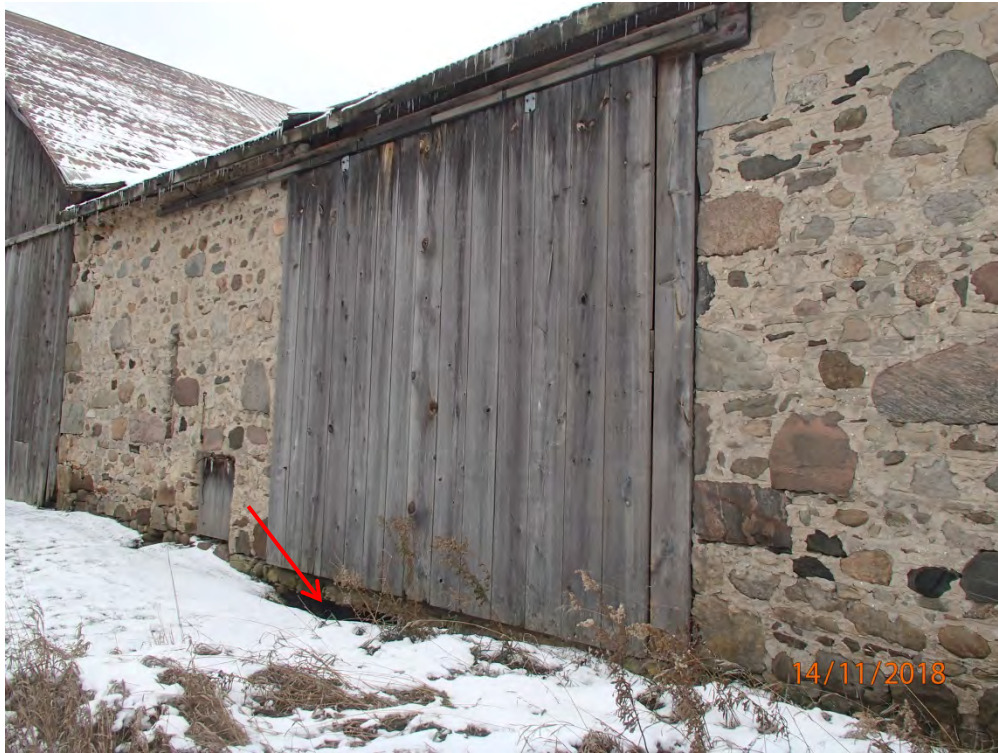
Photograph No. 1 – North wall at failed foundation wall.
