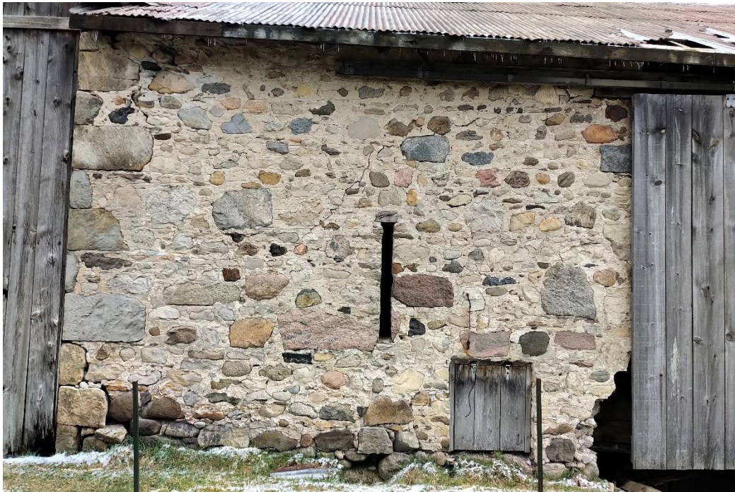
Photograph No. 8 – North Stone wall (upper) further Deterioration and loss
