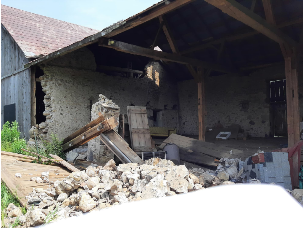
Photograph No. 1 – North Wall Collapsed – unsafe to shore
