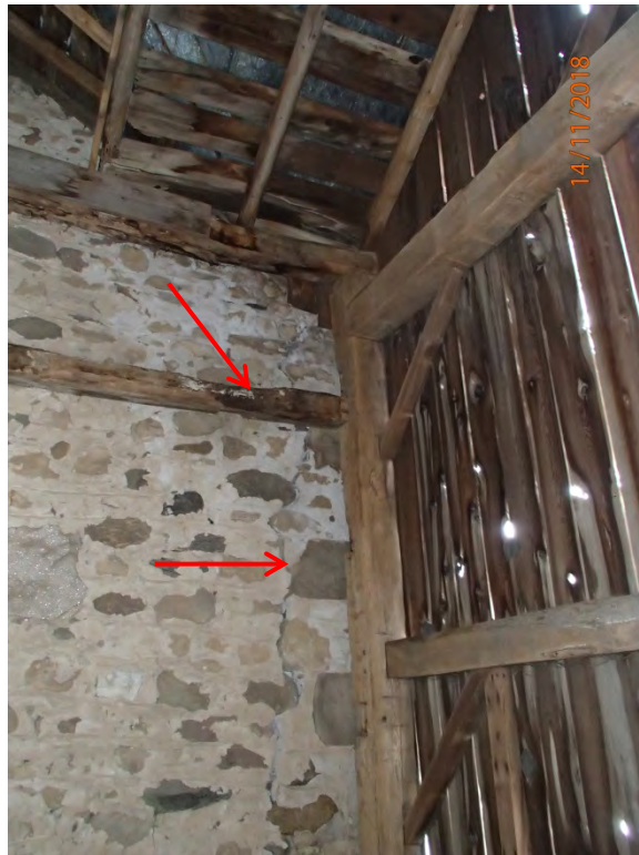
Photograph No. 6 – East Stone wall cracked, timber rot
