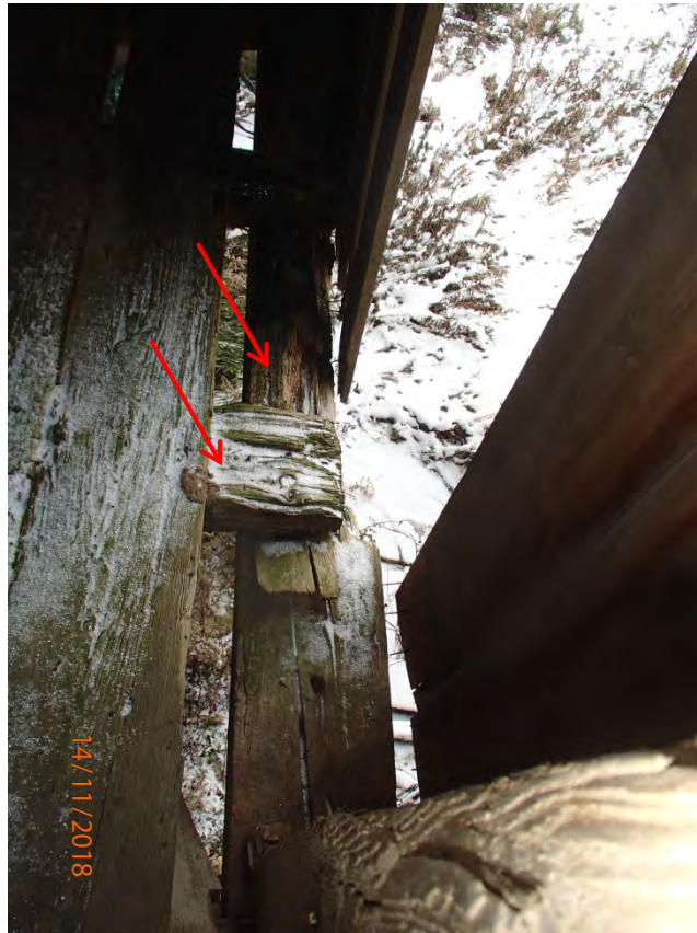
Photograph No. 14 – Rotted floor beam, potential fall hazard
