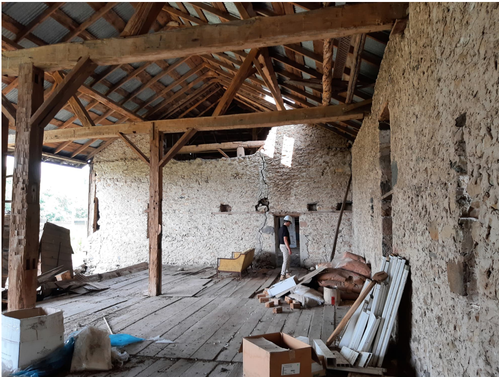
Photograph No. 6 – Stone Wall Cracked, Unsafe to work around
