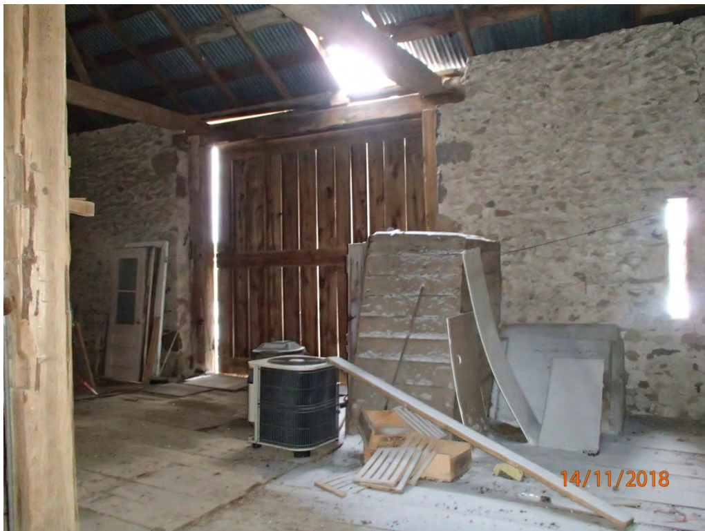
Photograph No. 5 – Door framing above failed foundation wall (interior view of north wall)
