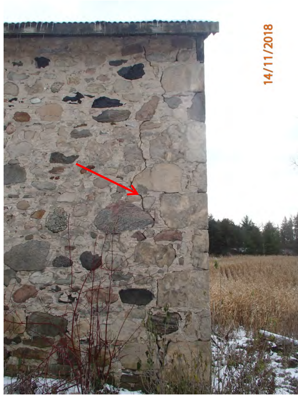
Photograph No. 18 – Northwest corner, thru crack in stone wall
