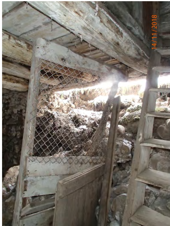
Photograph No. 3b – Failed foundation wall, floor beams unsupported
