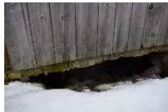
Plate 79: Collapsed foundation wall on north elevation
