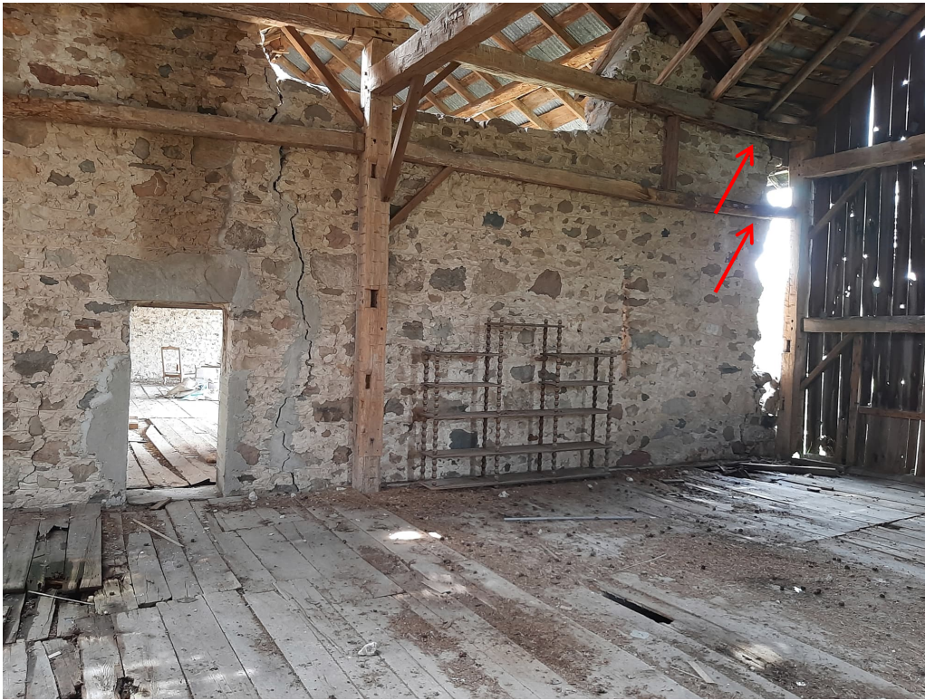
Photograph No. 7 – Stone Wall poorly braced at top – damaged timber (rot)
