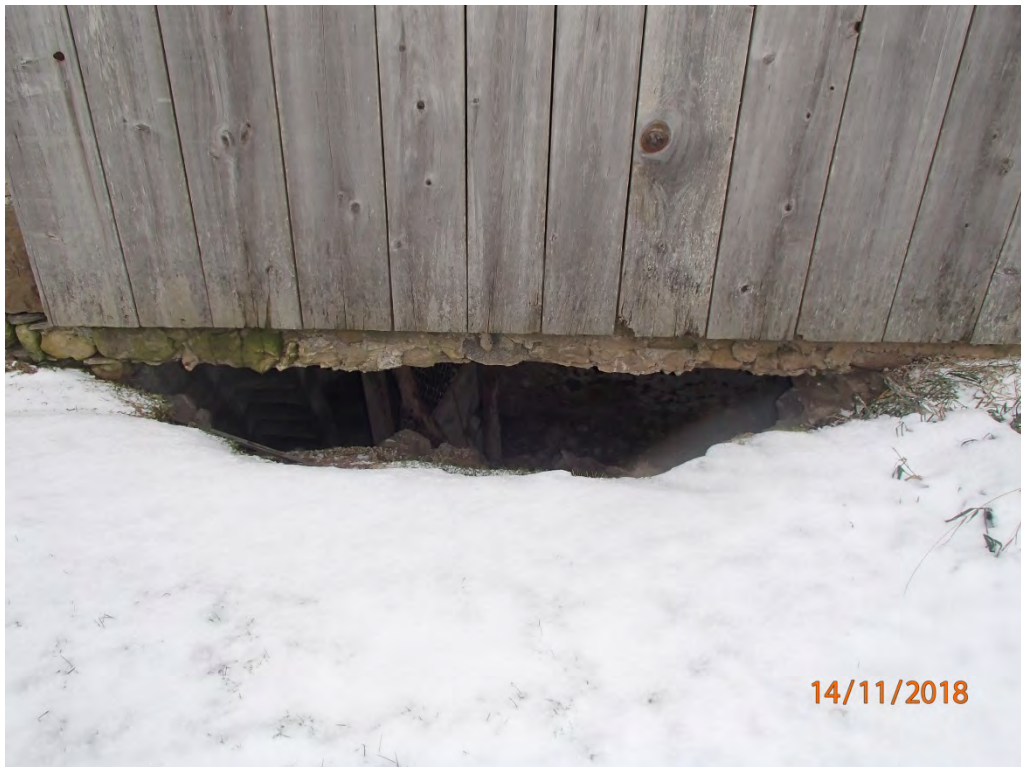
Photograph No. 2 – North foundation wall failure
