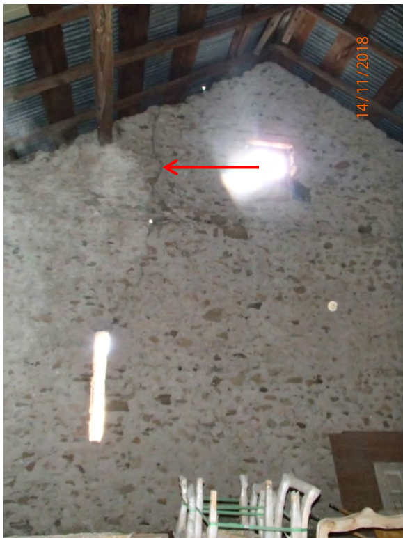
Photograph No. 8 – West Exterior Stone wall (interior view), cracked
