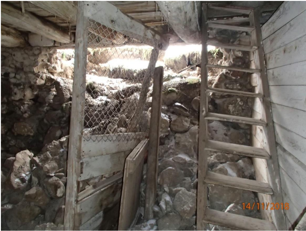
Photograph No. 3 – North wall (lower level) condition in 2018
