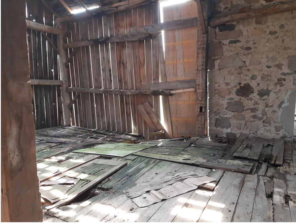
Photograph No. 9 – Southwest framing - floor and wall members compromised, unsafe
