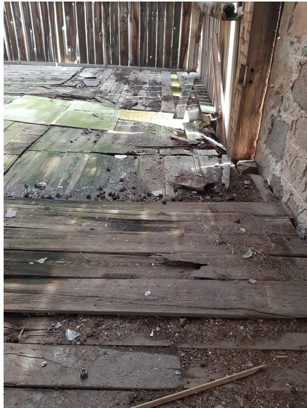
Photograph No. 10 – Floor and wall members compromised, unsafe
