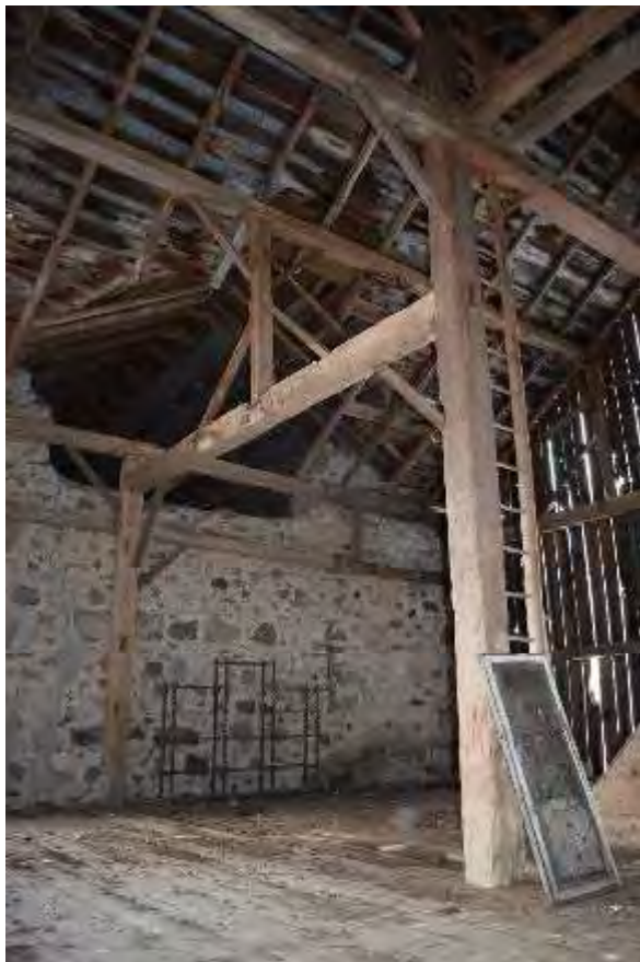
Plate 115: Stone tail east gable end looking northwest from timber frame portion of barn
