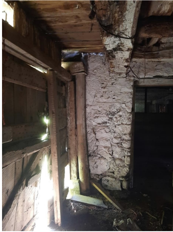
Photograph No. 11 – Structurally Compromised Floor Beam; Lower and Upper Posts vulnerable to collapse
