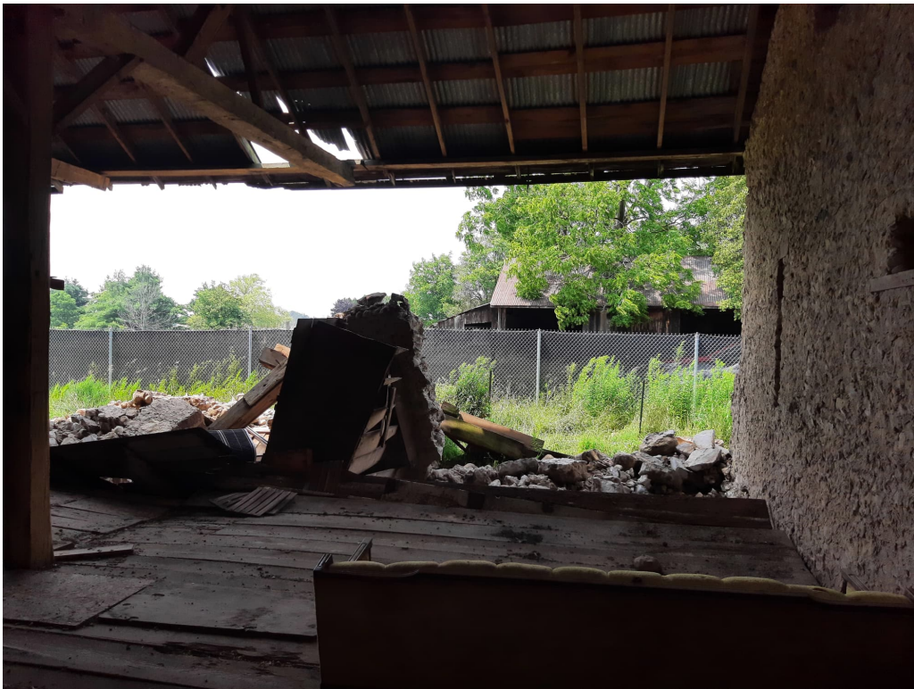
Photograph No. 2 – Unsafe to Shore or work under – Steel Roofing missing
