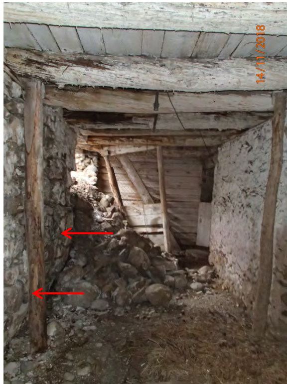
Photograph No. 4 – Bowing of North foundation wall
