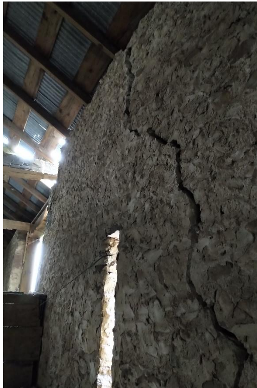
Photograph No. 10 – North wall (main floor) has moved in; crack worsened, opening up
