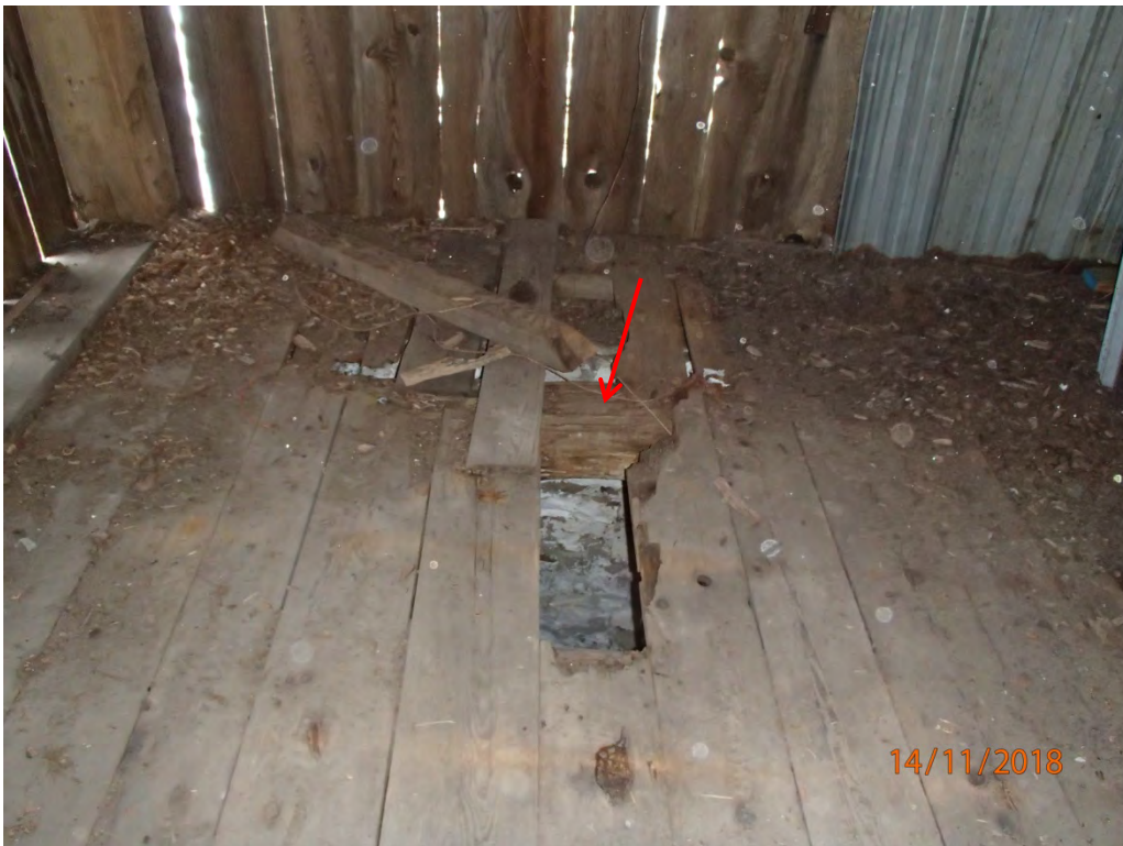
Photograph No. 11 – Unsafe floor boards, rotted floor beam
