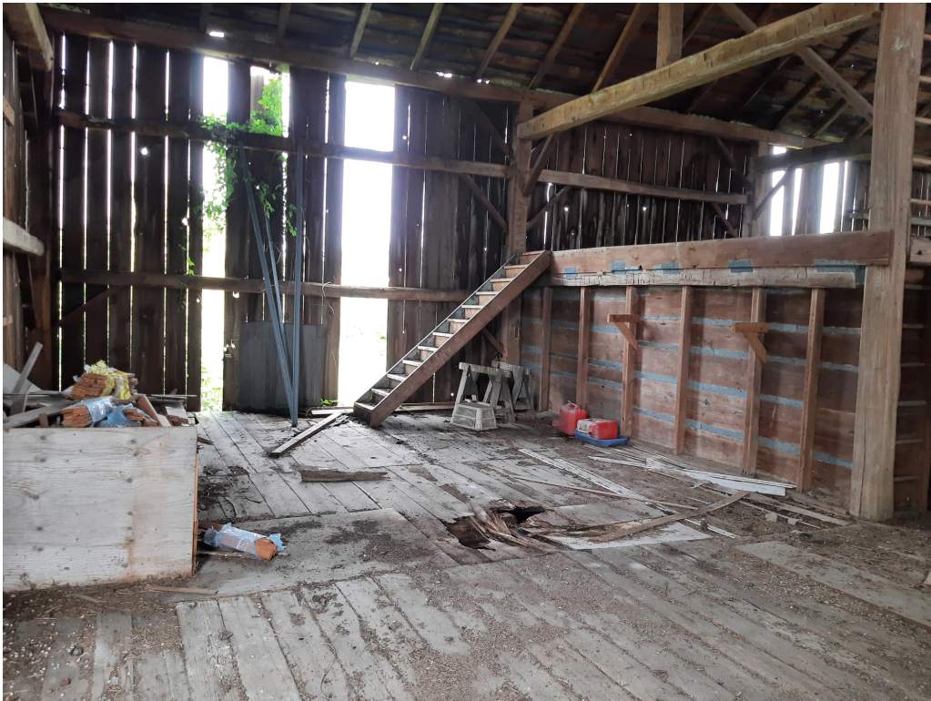
Photograph No. 14 – Floor, wall boards and framing unsafe
