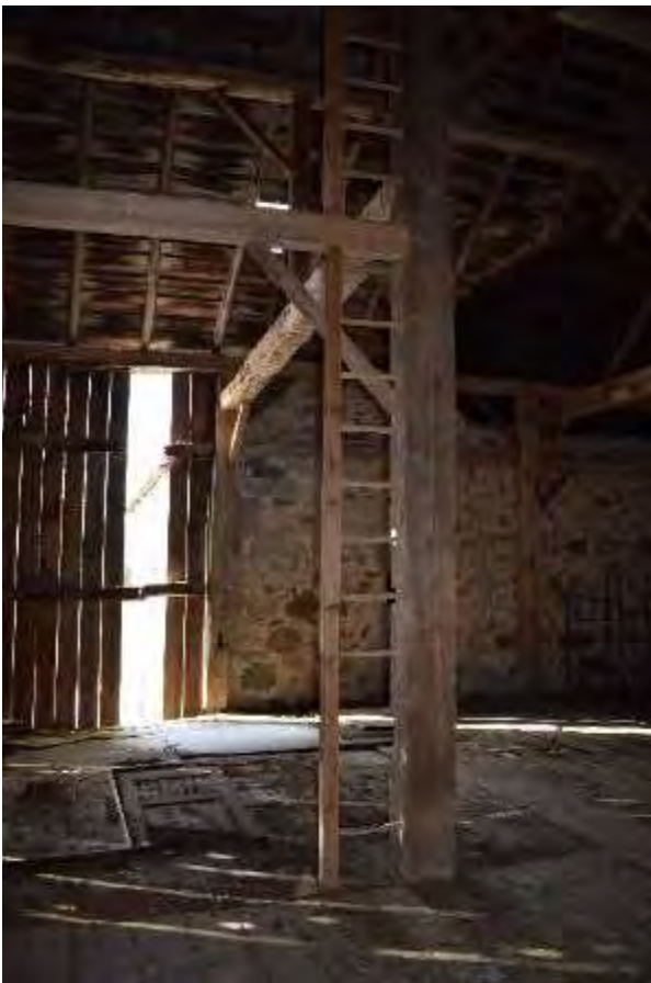
Plate 102: Wood ladder on interior post
