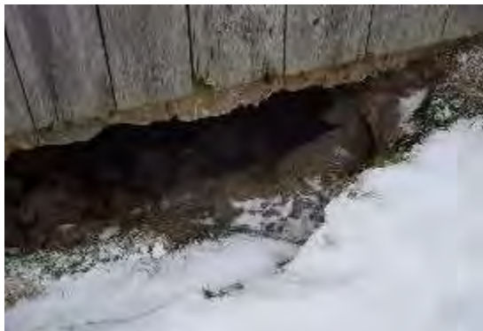
Plate 80: Close-up of collapsed north elevation foundation wall
