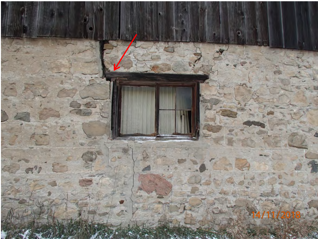
Photograph No. 23– Crack at lintel, inadequate bearing (south wall)
