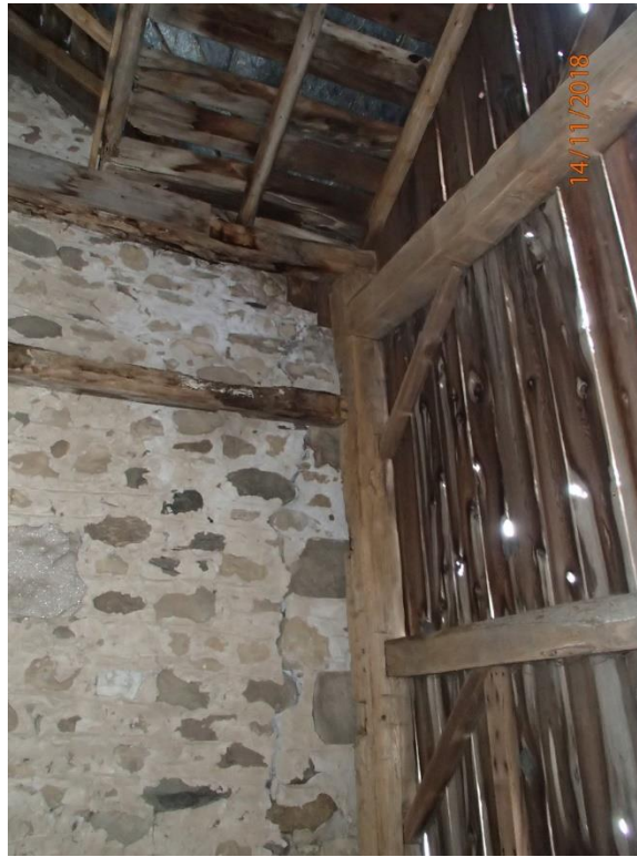
Photograph No. 11 – Crack interior, condition in 2018
