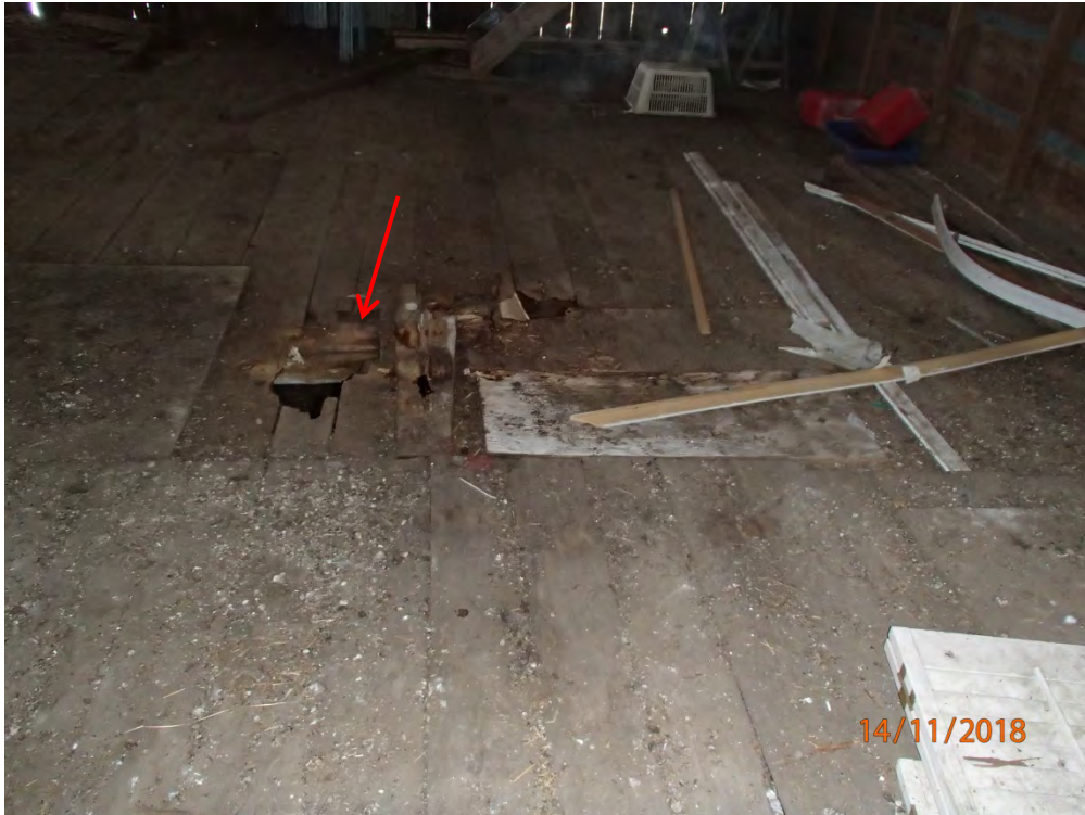
Photograph No. 10 – Unsafe, damaged floor boards
