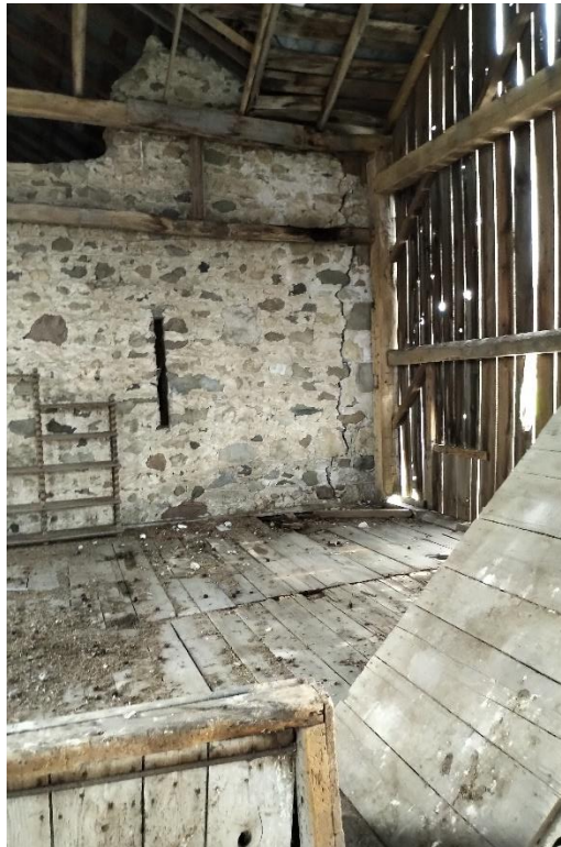
Photograph No. 12 – Crack opened wider due to north wall rotation inward
