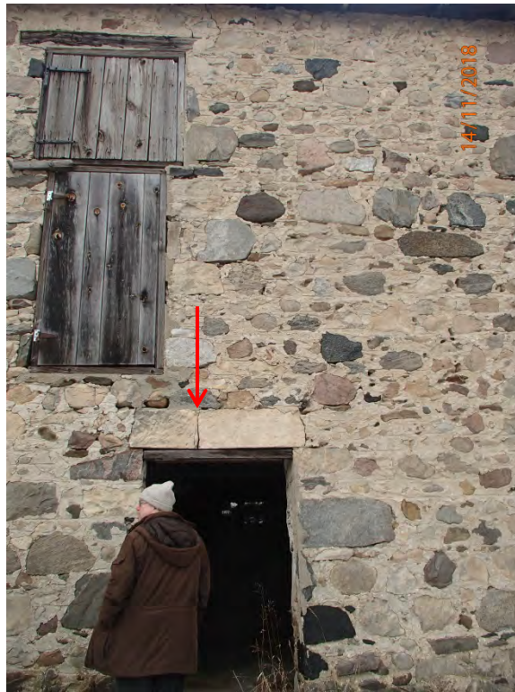
Photograph No. 16– Cracked lintel stones (South wall)
