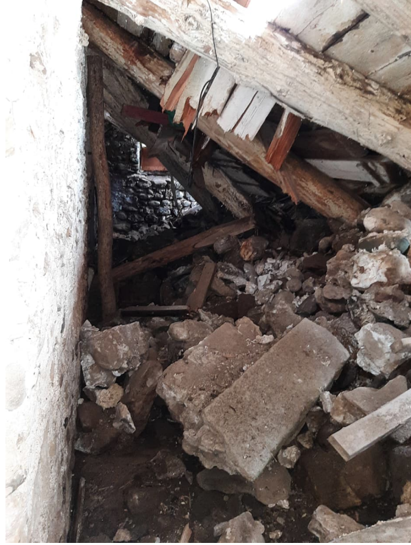
Photograph No. 5 – Collapsed North wall - unsafe to shore
