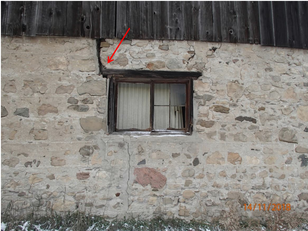
Photograph No. 18 – Crack at lintel, inadequate bearing (south wall)
