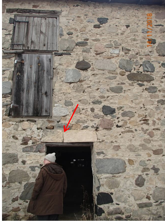
Photograph No. 15 – Cracked lintels (South wall)
