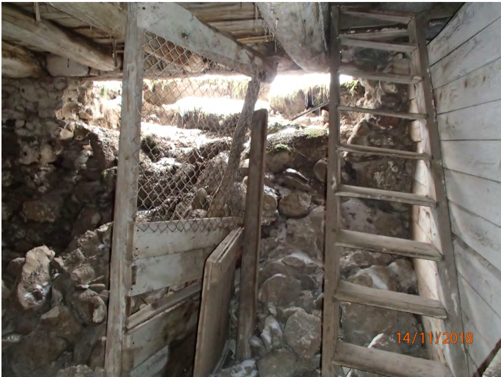
Photograph No. 3a – Failed foundation wall, floor beams unsupported
