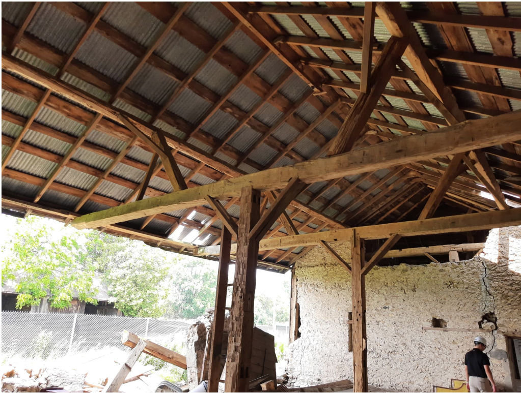
Photograph No. 3 – Damaged roof members; missing metal roof cladding
