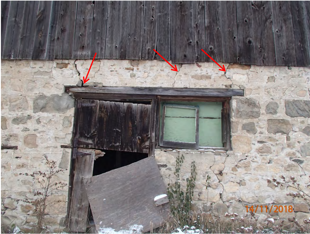
Photograph No. 22 – South wall, cracked stone over wood lintel
