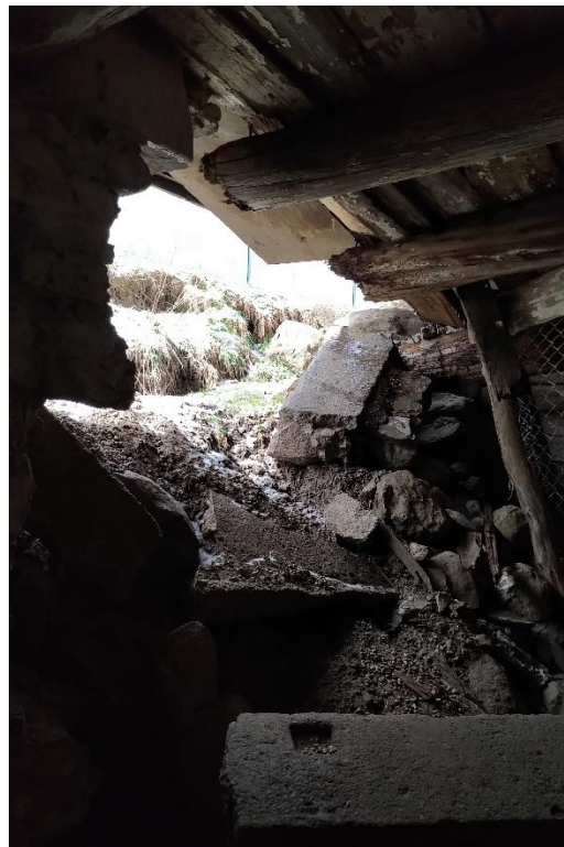
Photograph No. 6 – North wall (lower level – Left bearing) condition worsened: loss of more stone wall; floor support
