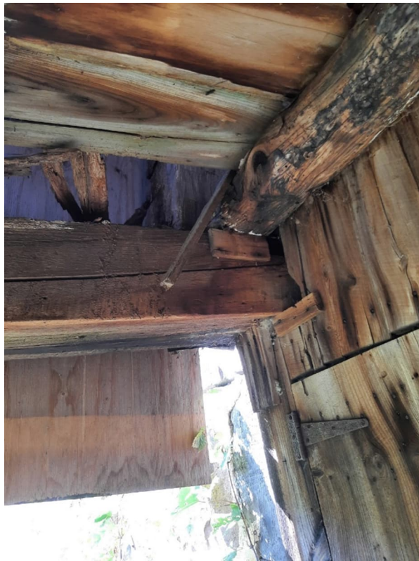
Photograph No. 12 – Floor beam cracked, sagging, unsafely supporting upper column
