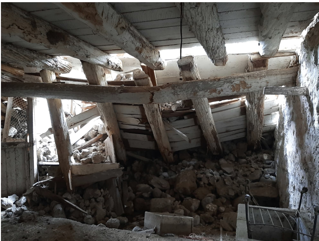
Photograph No. 4 – Collapsed North wall – unsafe to shore
