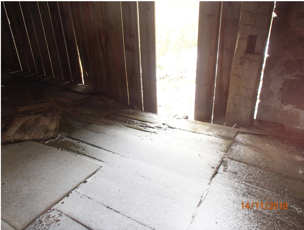
Photograph No. 8 – Taken 2018-11-14 - Condition worse today; floor and wall members compromised, unsafe
