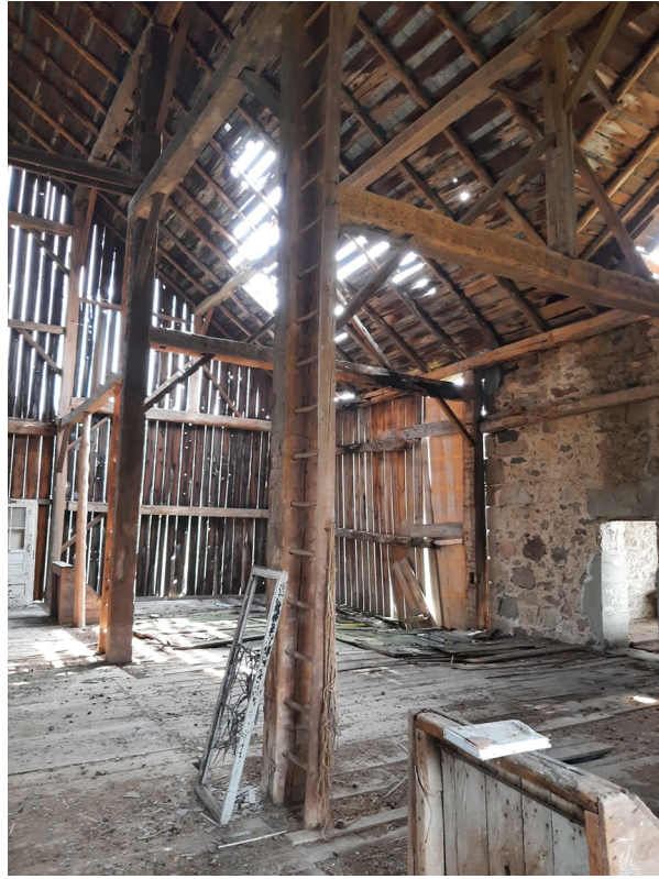
Photograph No. 13 – Unsafe to work on roof cladding
