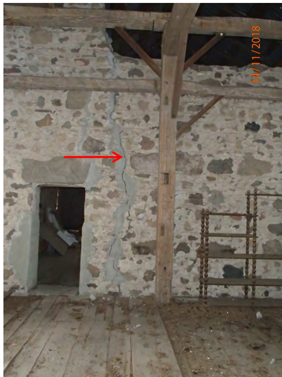
Photograph No. 7 – East Stone wall of Original Building (now interior wall), cracked
