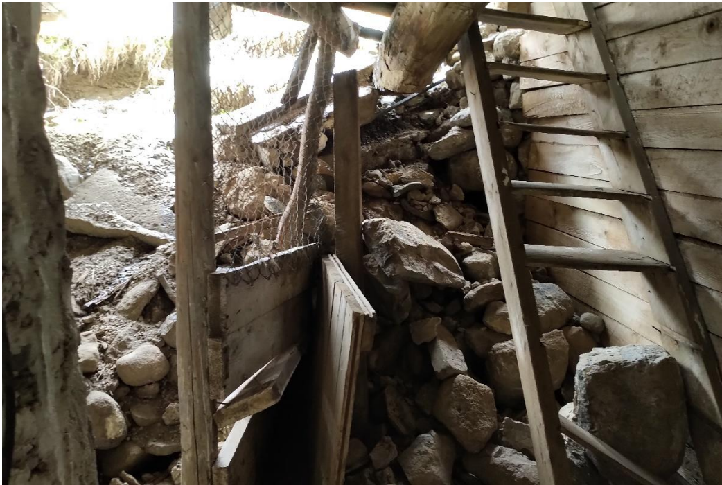
Photograph No. 4 – North wall (lower level) condition worsened: loss of more stone wall; floor support
