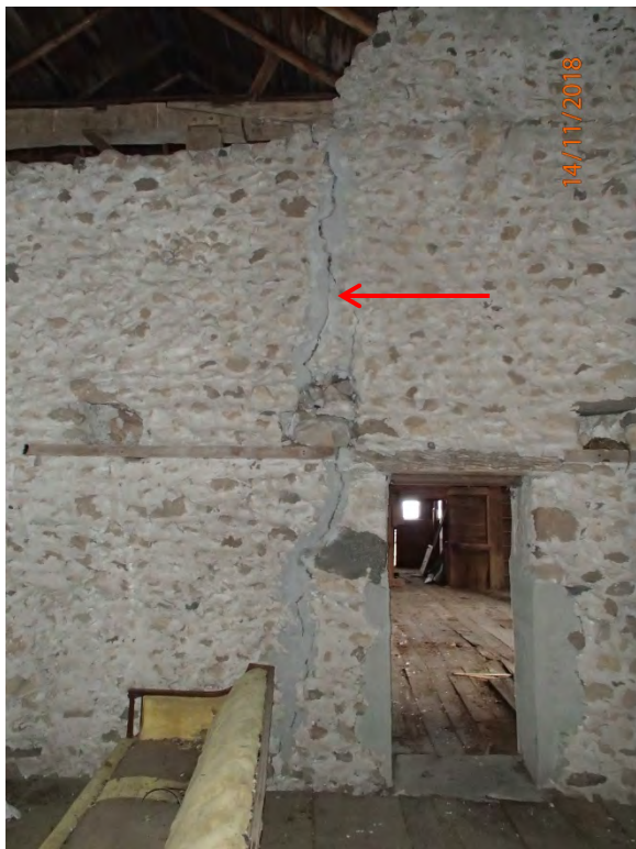
Photograph No. 9 – East Stone wall of Original Building (now interior wall), cracked
