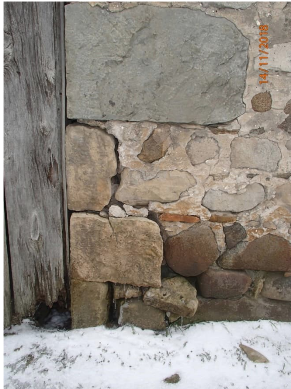
Photograph No. 16 – Stone wall mortar deterioration (North), rotted barn boards
