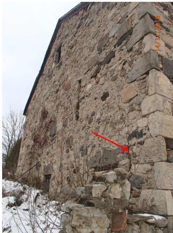
Photograph No. 17– West stone wall, cracks present but true (vertically plumb)
