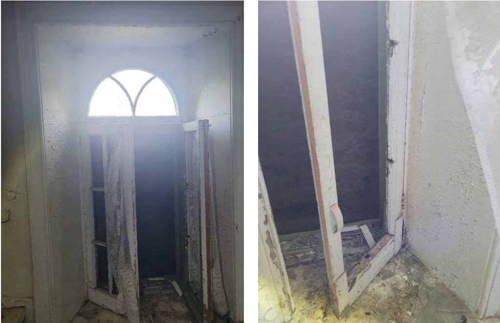
Figures 27 & 28: (left) Detail view of second storey central arched window noting broken glazing and wood frames (right) Detail of condition of wood window sash (Source: MHBC, 2023)
