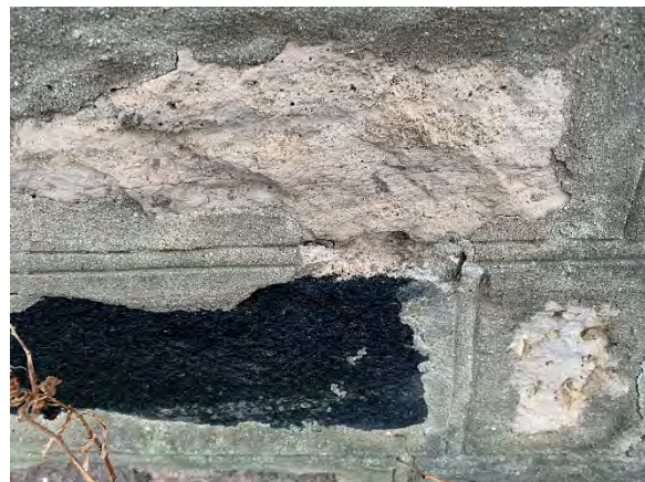
Photo 11: Typical Ashlar with Spalled Face and Tuck-pointing
