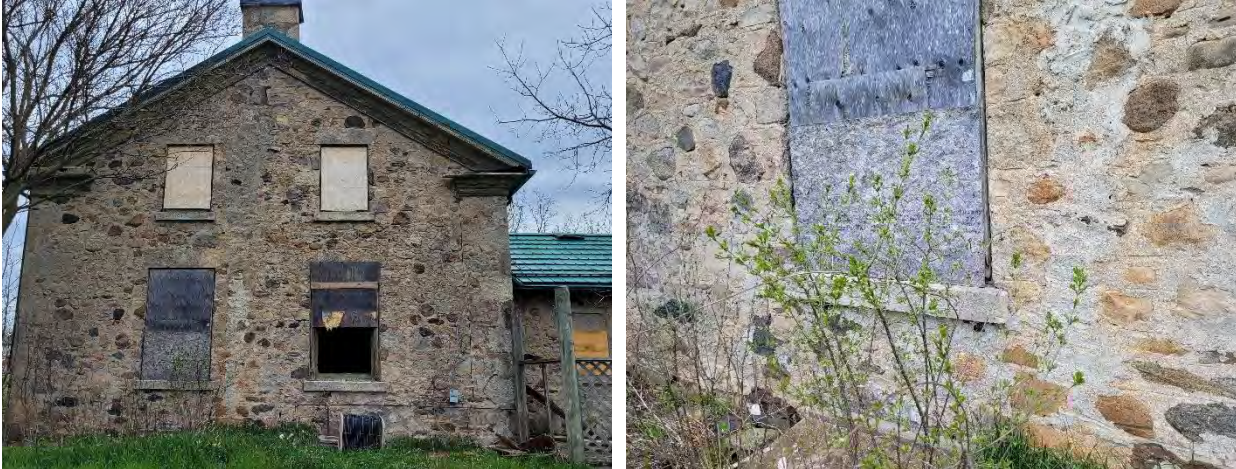
Figures 15 & 16: (left) View of north elevation, looking south (right) Detail view of broken window and sill at north elevation, (Source: MHBC, 2023)
