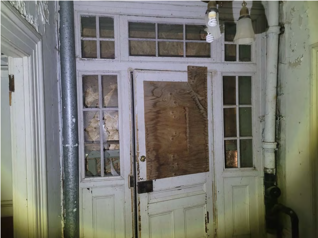
Figure 10: View of the original wood framed door, sidelights and transom (Source: MHBC, 2023)
