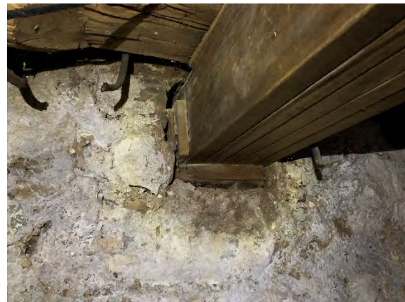
Photo 15: Typical Voids at Joist Ends
