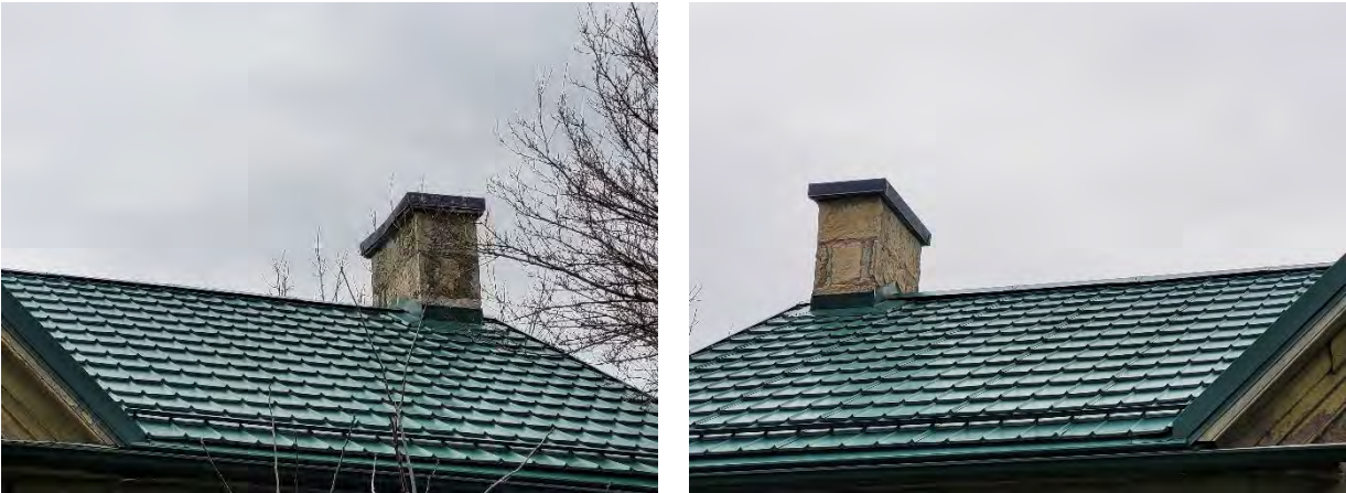
Figures 31 & 32: (left) View of roof noting chimney at south elevation (right) Detail of stone chimney located at south elevation (Source: MHBC, 2023)
