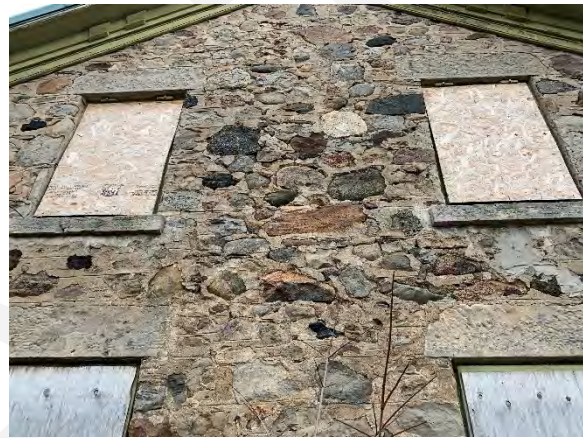
Photo 13: Washed-out mortar and loose stones in Rubble Wall
