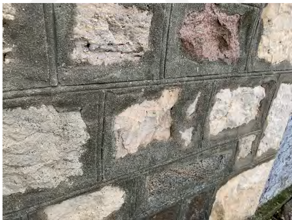
Photo 10: Typical Ashlar with Spalled Face and Tuck-pointing
