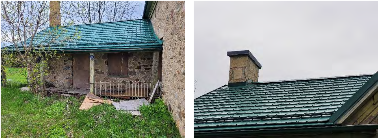
Figures 29 & 30: (left) View of roof, north elevation of Section "B" (right) Detail of condition of metal roof, Section "A" looking east from west elevation (Source: MHBC, 2023)
