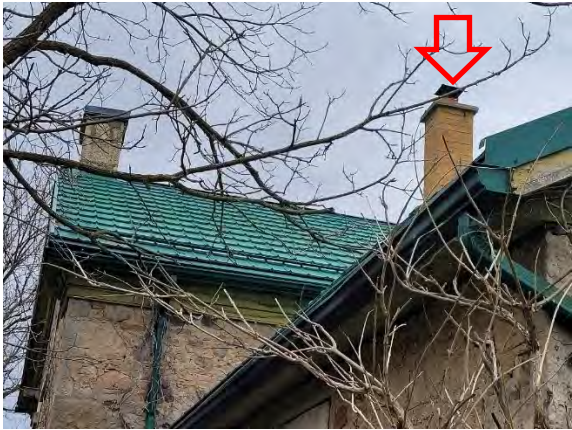
Figure 33: Detail of east elevation noting location of yellow brick chimney, Section "A" (Source: MHBC, 2023)
