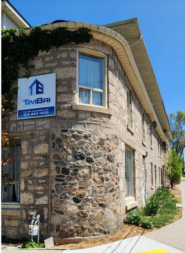
Figure 4 - Rounded corner at Gordon St and James St E; (Right) stone parapet marks earlier north wall. (Photo: S. Robinson, 2023)
