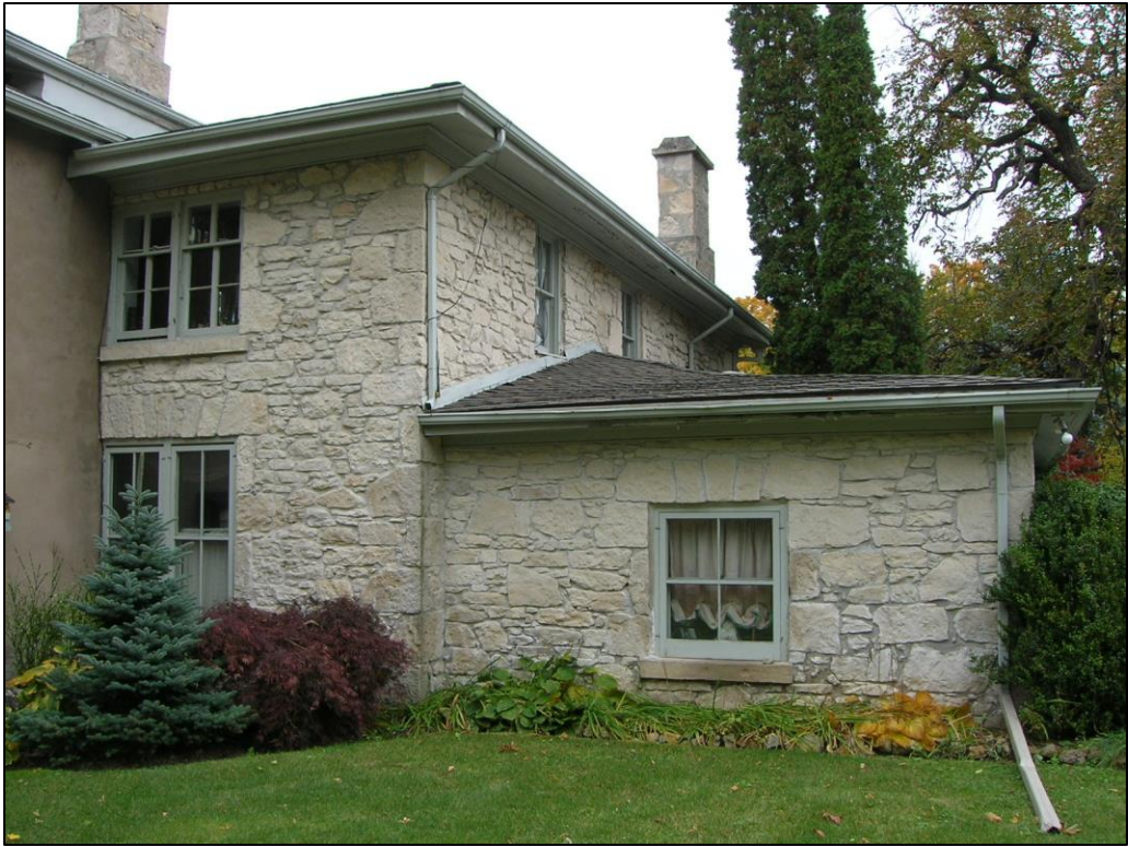
Figure 4: Northwest side of building, original limestone façade. Source: Site Visit with Franco Valeriote, 2009.
