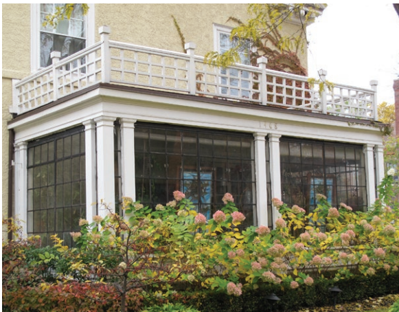
Residential porch enclosure set behind white rectangular columns, with black frames and mullions, Detroit, Michigan (Photo by Scott Weir).
