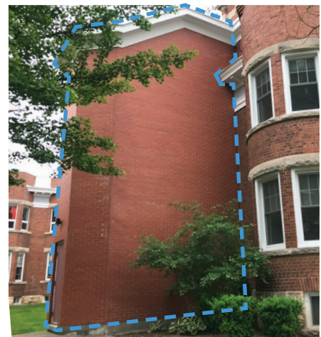
View of central wing within north courtyard indicating existing stairwell to be removed (ERA, 2024).
