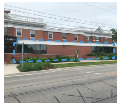
East elevation indicating area of non-original addition to be re-clad in blue (ERA, 2024).
