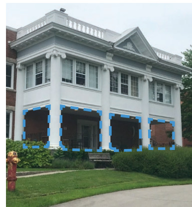
North and west elevations of north portico, indicating areas to be enclosed in blue (ERA, 2024).
