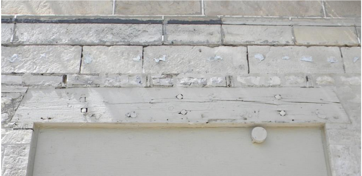
Figure 5: Wooden lintel on main floor, possibly from the 1840's stable building. The opening is similar in size to the ones visible in the photographs from the 1880s. (Photo: S. Robinson, Heritage Planning)
