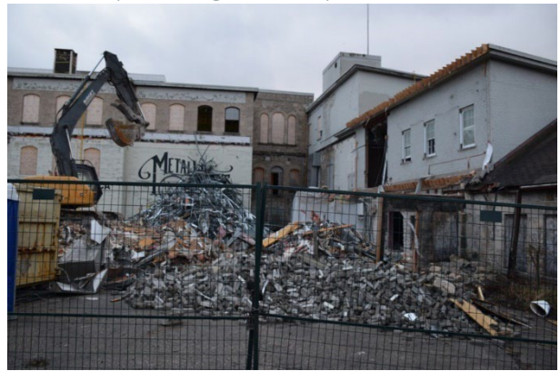
Figure 37: Site of the former W. C. Wood Company during the demolition process, with elements of the former industrial complex being retained (O’Flanagan, 2016)
