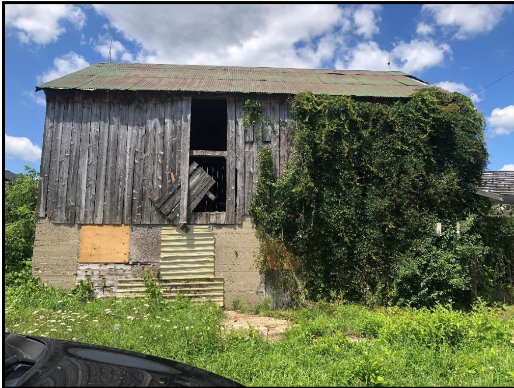
Image 11: 316 Grange Road – Timber Barn Façade (Southeast Elevation) (Photo taken July 22, 2025; Facing Northwest)
