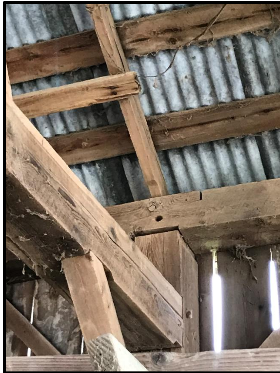
Image 41: 316 Grange Road – Upper Floor, Mortise and Tenon Joinery Secured by Wooden Pegs (Photo taken July 14, 2021)
