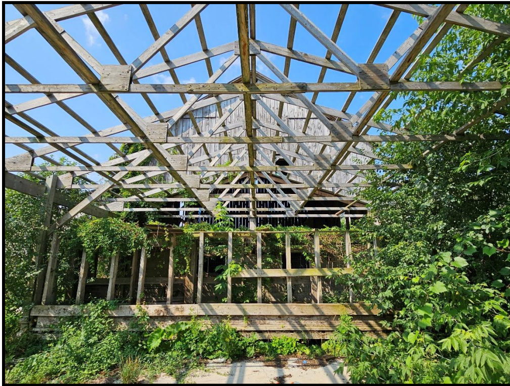
Image 27: 316 Grange Road – Timber Barn Wood Frame Addition Interior (Photo taken July 22, 2025; Facing Southwest)
