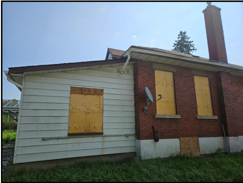
Image 5: 316 Grange Road – Residence Southwest Elevation (and Rear Addition) (Photo taken July 22, 2025; Facing Northeast)
