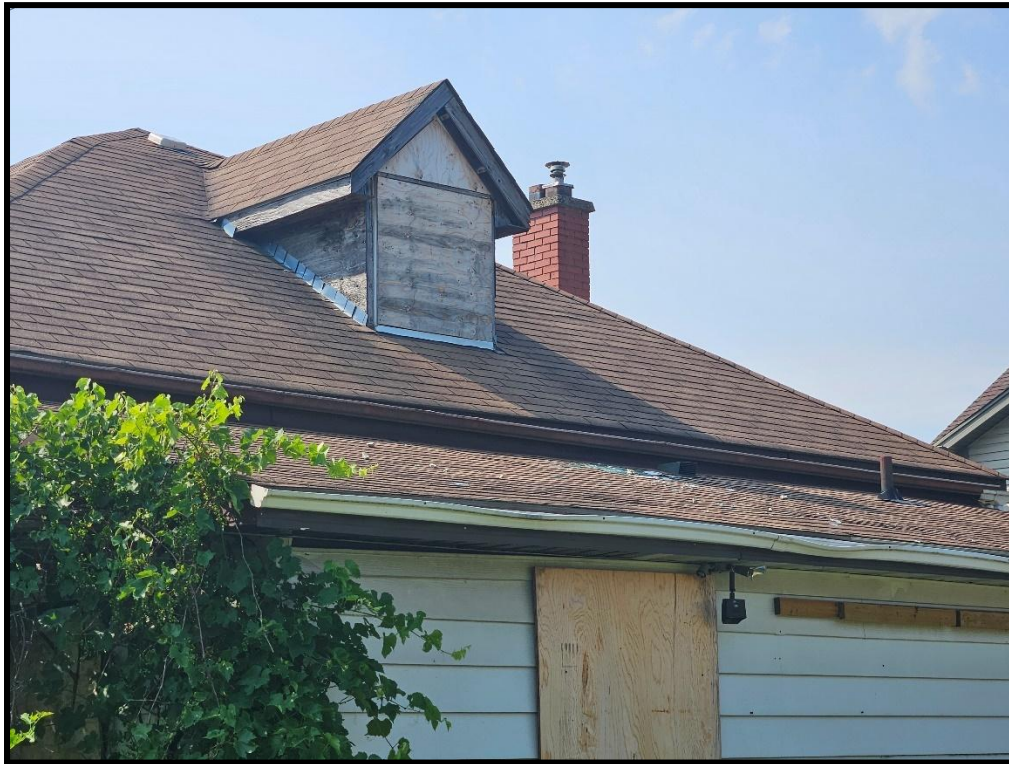
Image 9: 316 Grange Road – Residence Rear Addition Gable Window (Photo taken July 22, 2025; Facing South)
