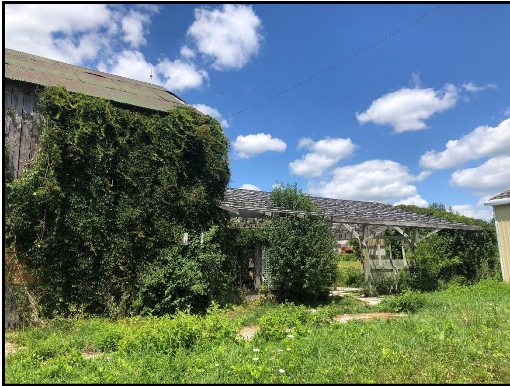
Image 25: 316 Grange Road – Timber Barn Wood Frame Addition (Photo taken July 22, 2025; Facing North)
