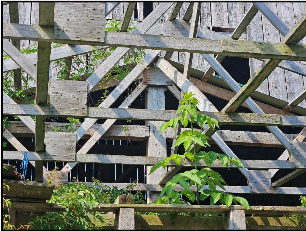
Image 29: 316 Grange Road – Detail of Timber Barn Wood Frame Addition Truss (Photo taken July 22, 2025; Facing Southwest)
