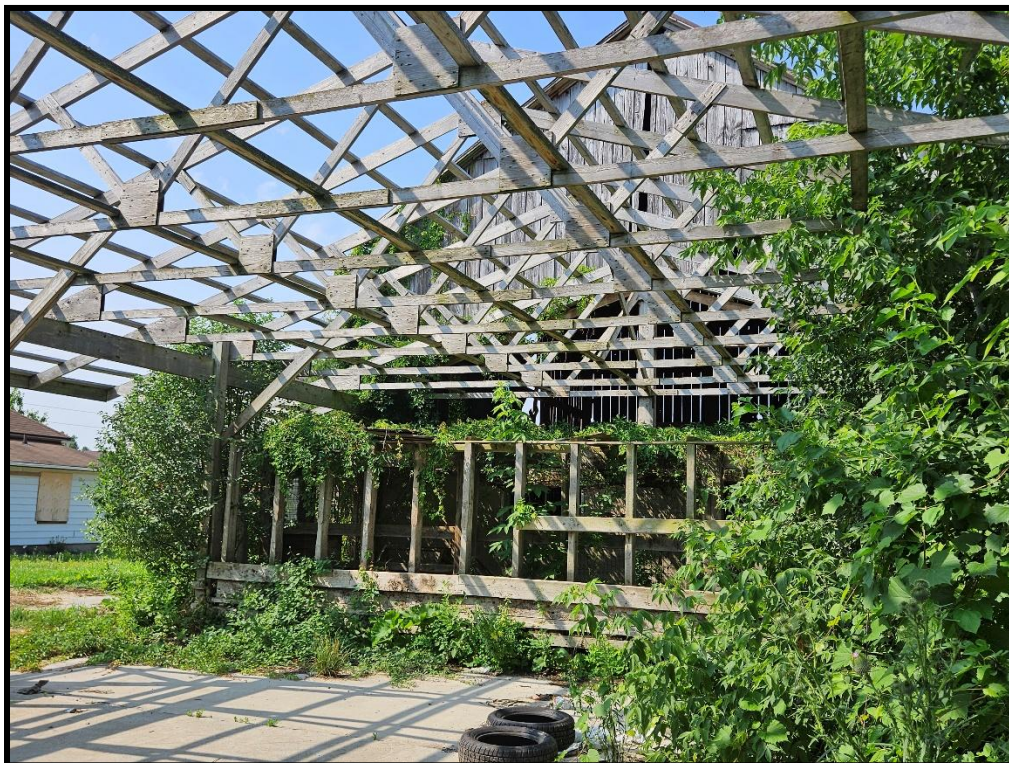
Image 30: 316 Grange Road – Timber Barn Wood Frame Addition (Photo taken July 22, 2025; Facing Southwest)
