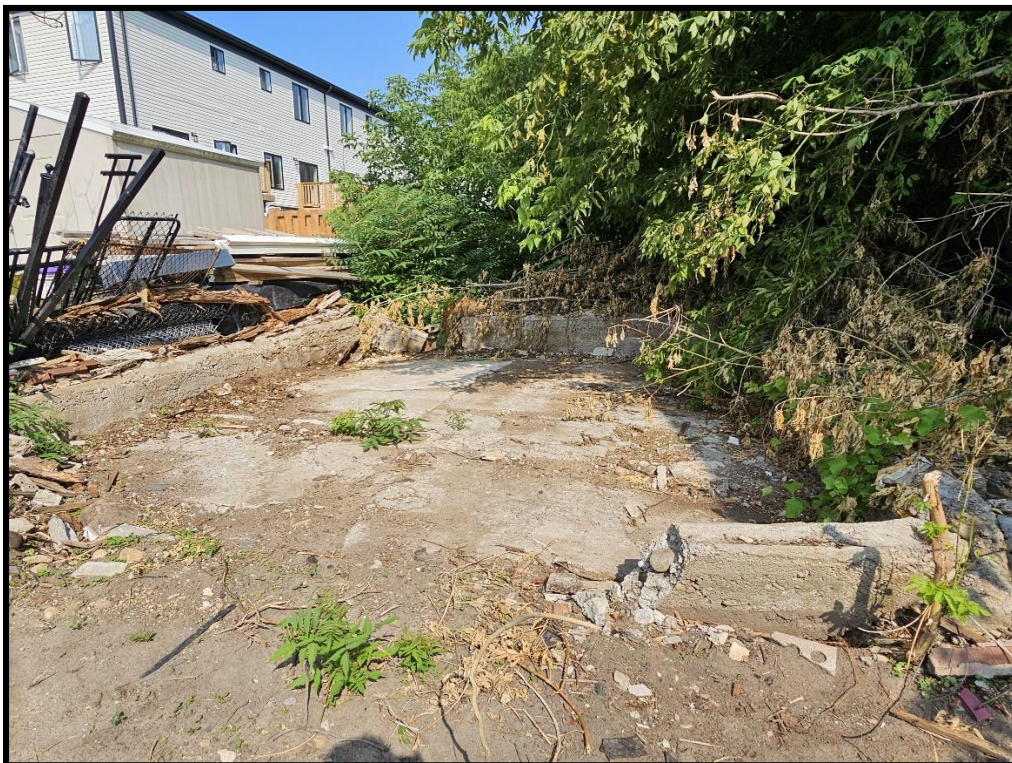
Image 38: 316 Grange Road – Concrete Pad, Site of Former Outbuilding (Photo taken July 22, 2025; Facing Northwest)
