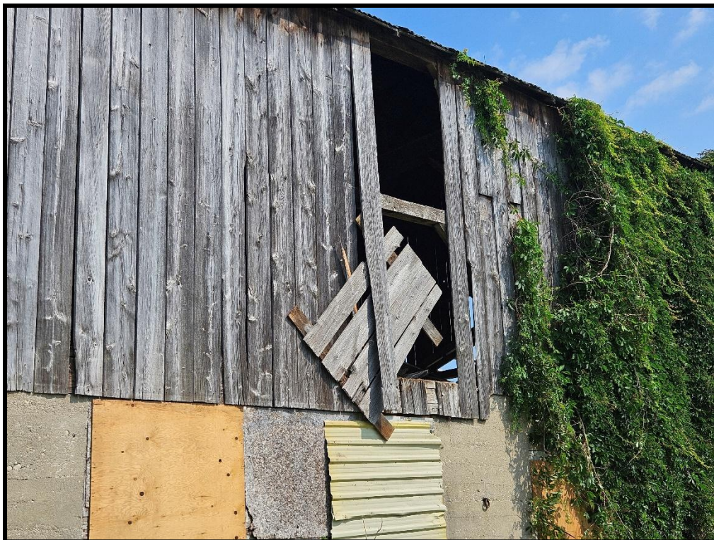
Image 12: 316 Grange Road – Timber Barn Detail of Missing Vertical Barn Boards (Photo taken July 22, 2025; Facing North)
