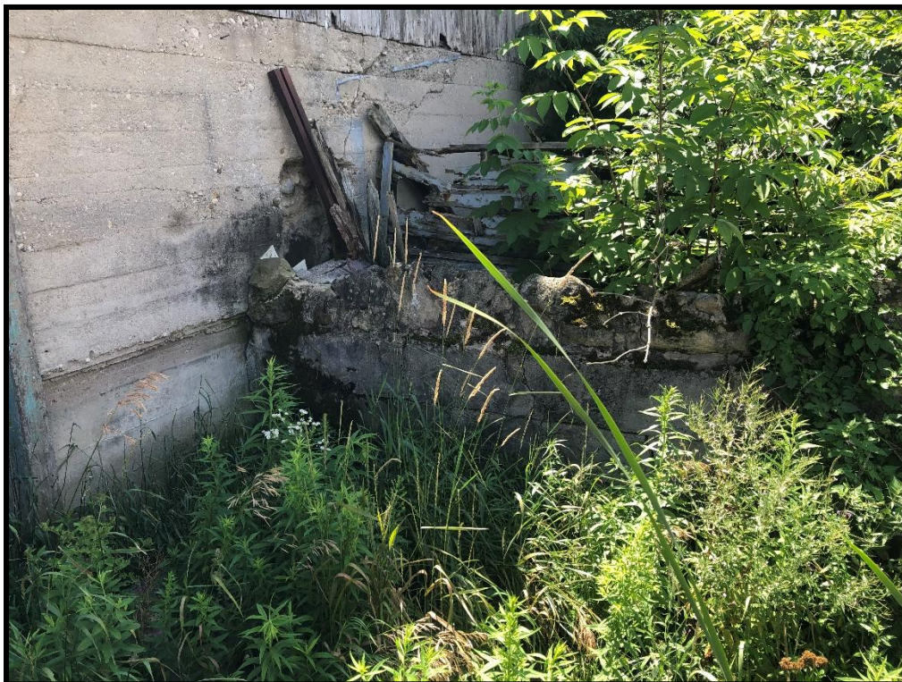
Image 22: 316 Grange Road – Timber Barn Stone and Concrete Walls (Photo taken July 22, 2025; Facing Southwest)
