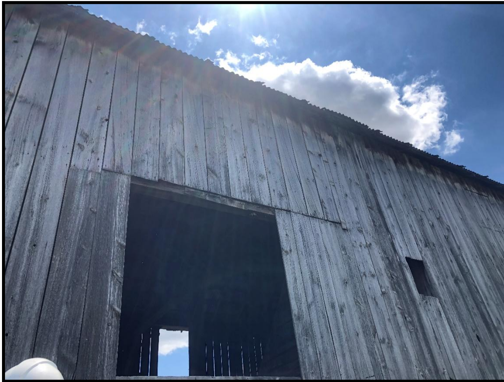
Image 21: 316 Grange Road – Timber Barn Northwest Elevation Opening (Photo taken July 22, 2025; Facing Southwest)
