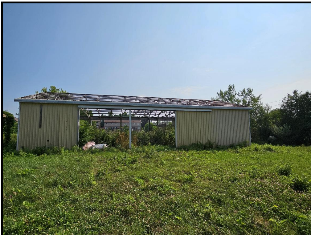
Image 32: 316 Grange Road – Steel Outbuilding Façade (Southwest Elevation) (Photo taken July 22, 2025; Facing Northeast)
