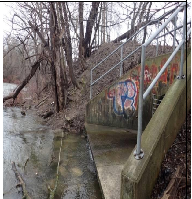
Photo F: Upstream section - left bank erosion at concrete spillway (image taken during high flow event)
