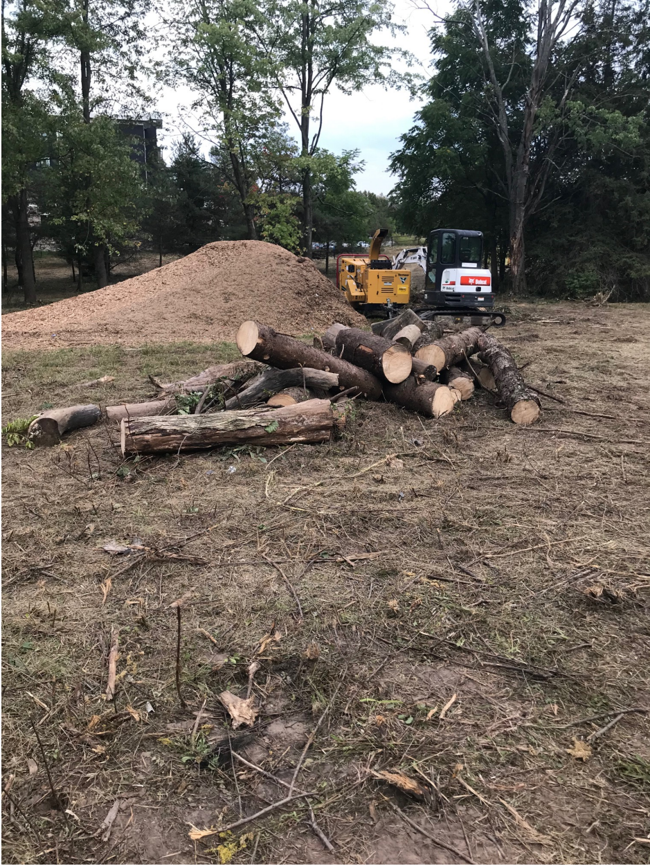
Trees which were removed by TriCar in preparation for the application to develop the land.
