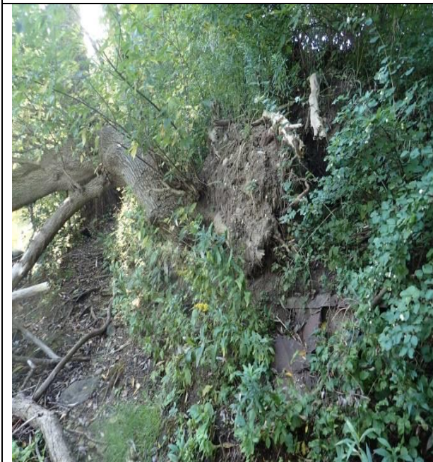
Photo E: Upstream section left bank erosion
